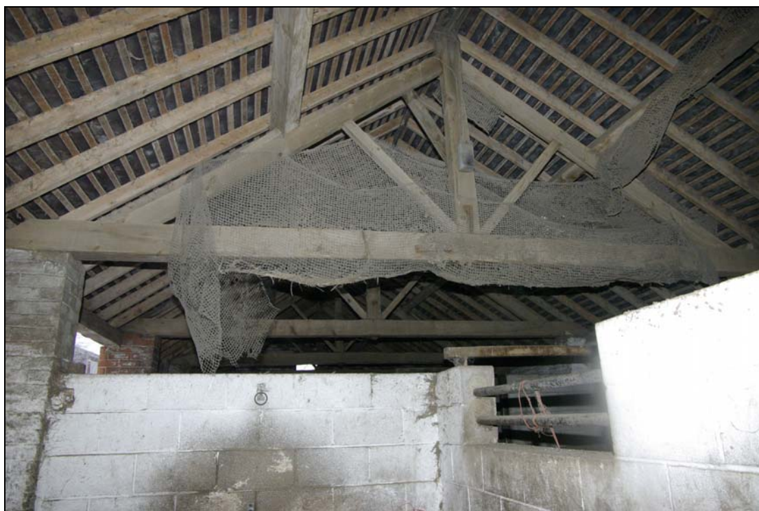
Plate 18. Range B, king-post roof truss over 19th century cow-shed, with breeze block walls forming 20th century stable conversion. Looking south-east.
