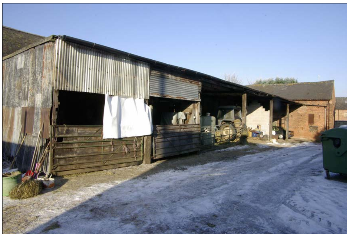
Plate 19. 20th century lean-to structures adjacent to Range A, Barn 1. Looking north, with Barn 2 in background.
