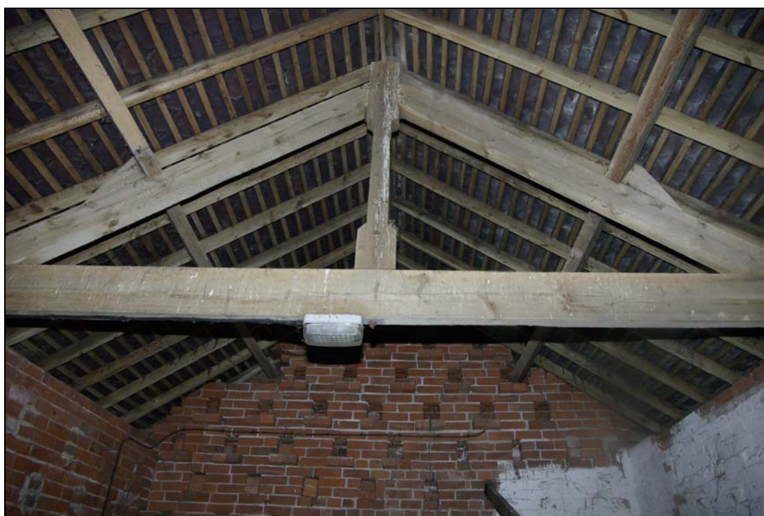
Plate 17. Range B, king-post roof truss and nesting boxes within two-storey stable block and hayloft. Looking south-east.
