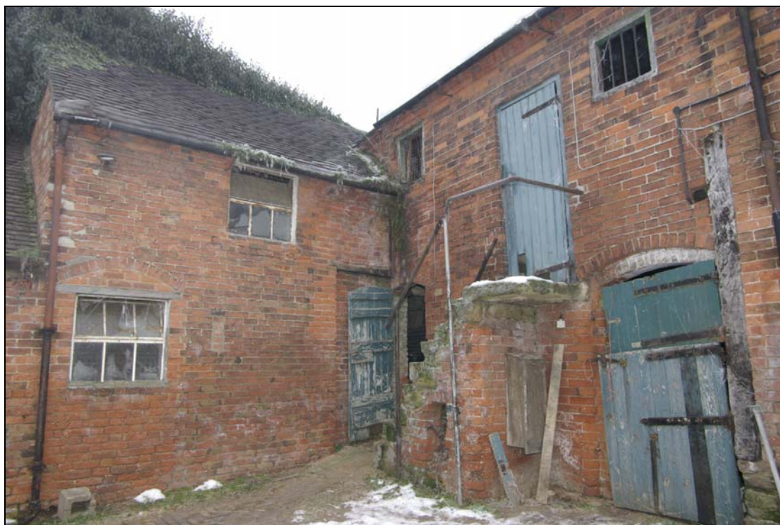
Plate 5. Junction of Barn 1, central store and cow-shed. Looking north-east, with timber post relating to early structure visible on right.
