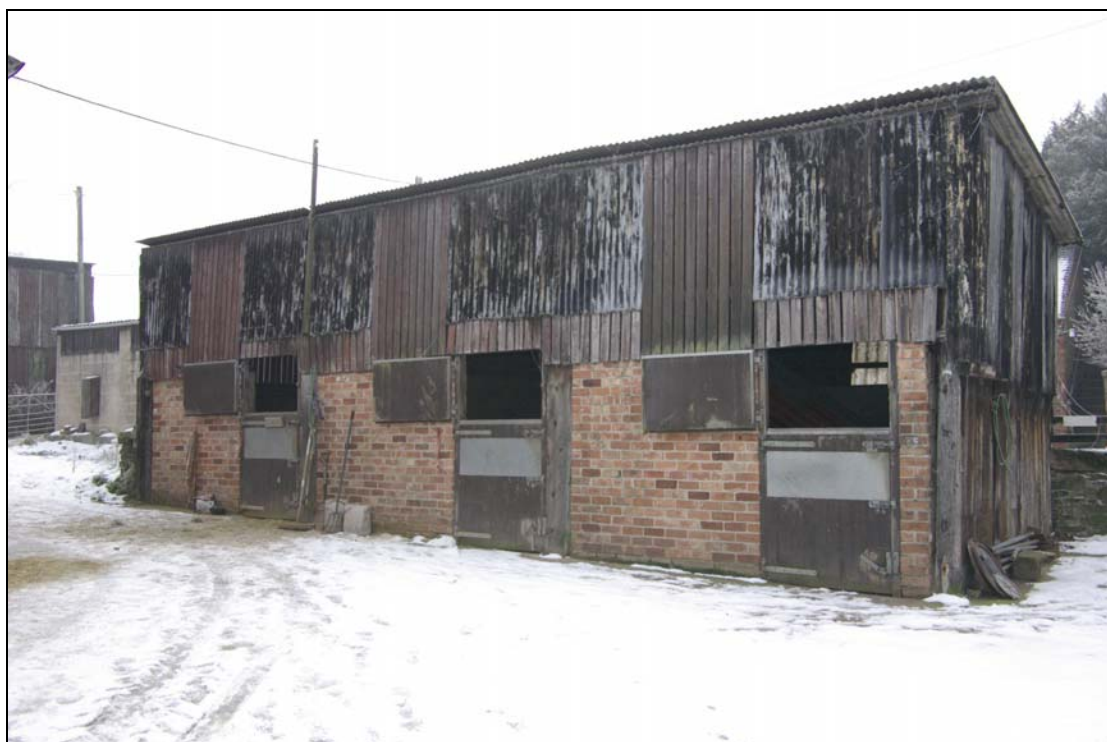
Plate 21. 20th century brick and timber stable block located within foldyard. Looking south-east.
