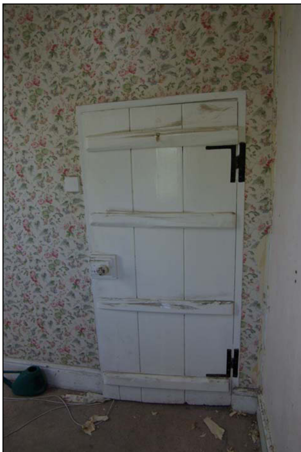
Plate 11. Late C17th plank and batten door, with L-hinges. Re-used in bathroom within 1850+ range. Looking south-east.
