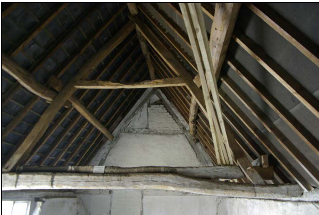
Plate 13. Early C18th outbuilding, first floor. Principal roof truss, with purlins pegged through back of principals. Looking south-east.
