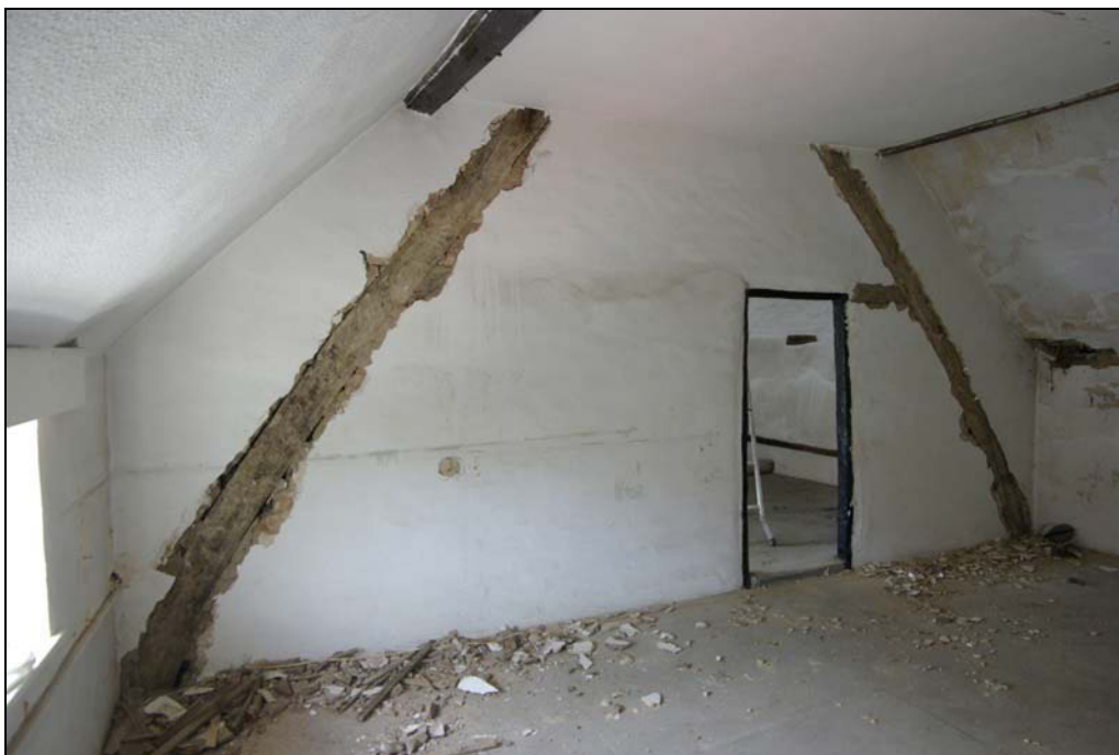
Plate 9. Cruck blades of upper-cruck truss, revealed behind plasterwork. First floor, looking west.
