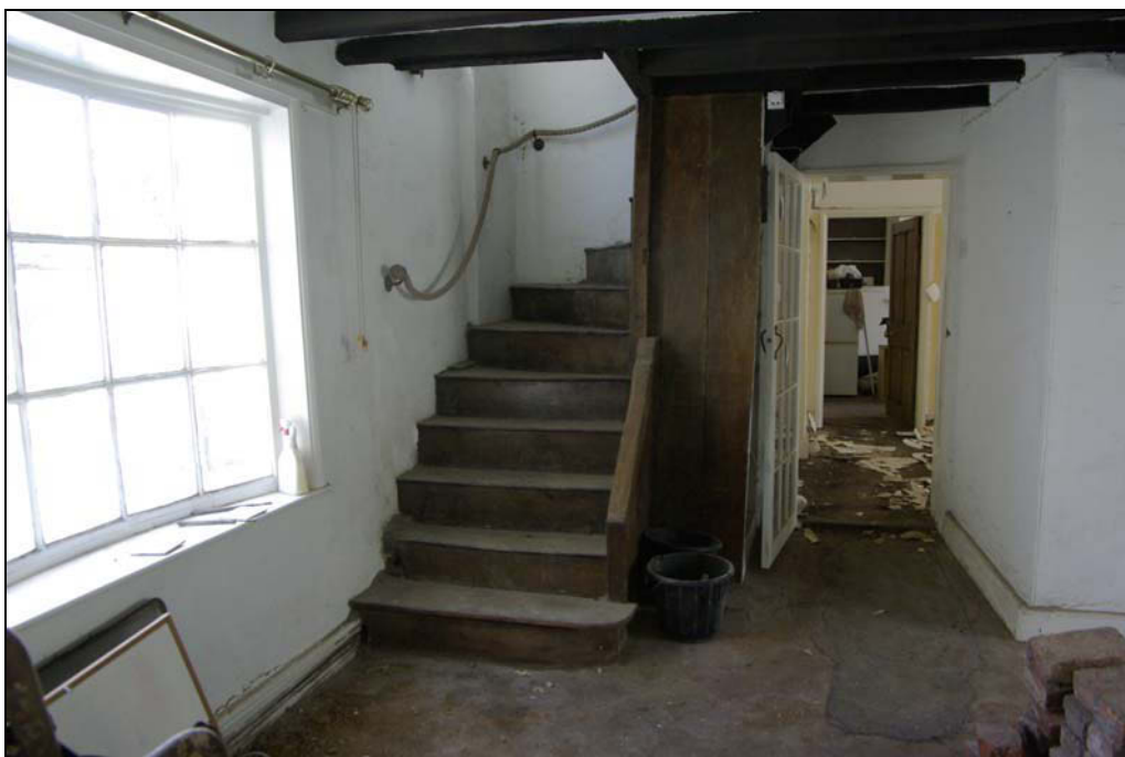
Plate 6. Late C17th staircase, with trimmers pegged into the ceiling joists. Looking north-east.
