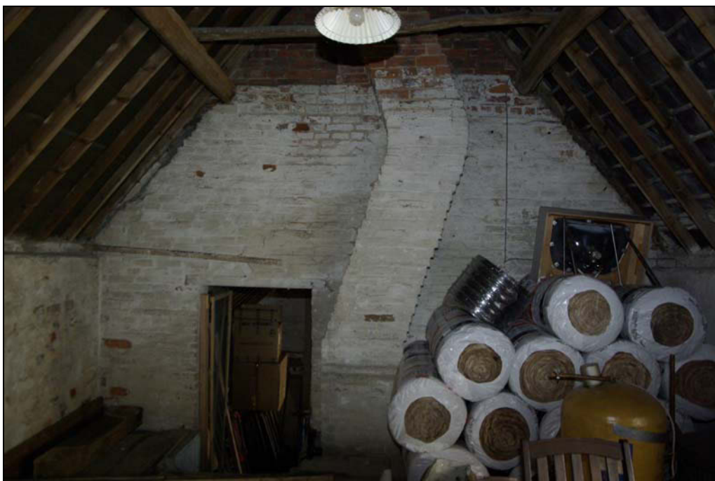
Plate 14. Early C18th outbuilding, rebuilt gable with inserted, cranked chimney stack. Looking north-west.
