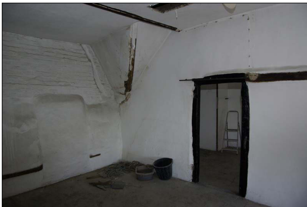
Plate 12. Junction of late C17th house with early C18th outbuilding and inserted (blocked) doorway through. Looking north.
