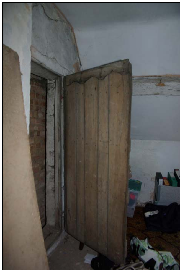
Plate 15. 18th century plank and batten door with decorative fascia board. 20th century brickwork skin to exterior of northern gable end visible through doorway. Looking east.
