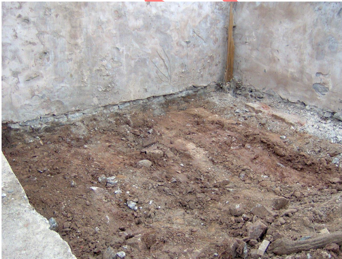
Figure 6 Area of lifted slab.
