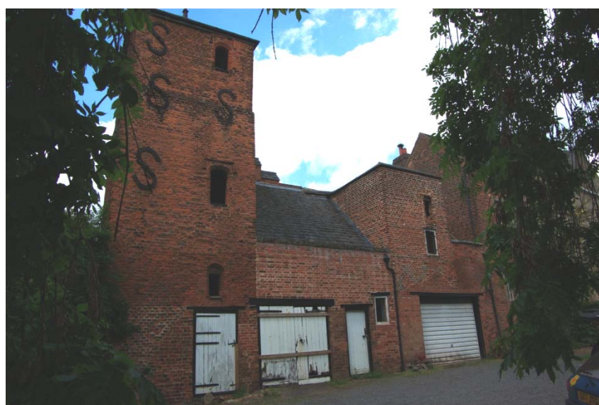
Photo. 3. Late 15 th century brick towers (Range B to left & C to right) from the SW
