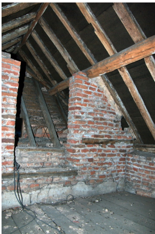
Photo. 7. Attic room Range E with steps down from blocked entrance in Range G
