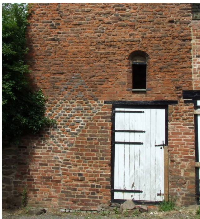
Photo. 5. Truncated diaper work and inserted door in south-east elevation of tower B
