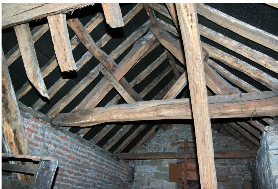
Photo. 13. Attic room Range H, showing roof truss (identical to that in Range F)
