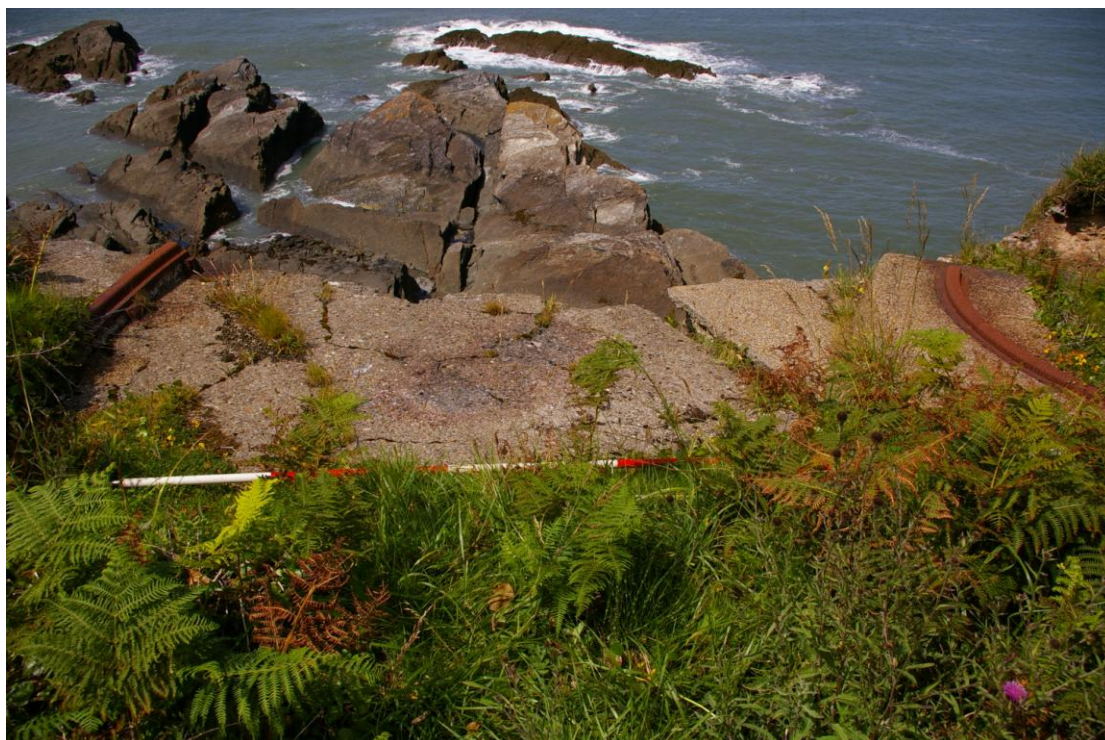
Figure 11: 56279; Gun Battery from south. The cast iron tracks are at 3.90m centres, although this has been widened by cracking in the concrete on which they are set. A low retaining wall lies on the right hand side. The structure is eroding over the cliff edge.
