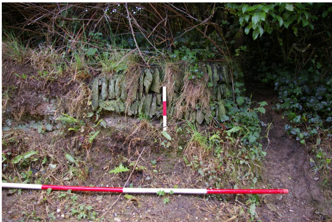
Figure 24: Observation 2, retaining wall from west on eastern edge of coastal path. The wall is L shaped in plan with a return on the southern side.
