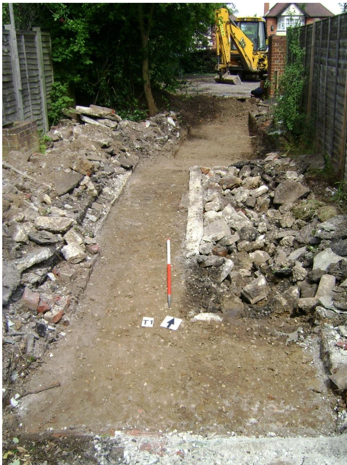
Figure 7. Trench after initial 10 metre excavation Looking north-west, 1m scale. Backfilled pond on right of picture
