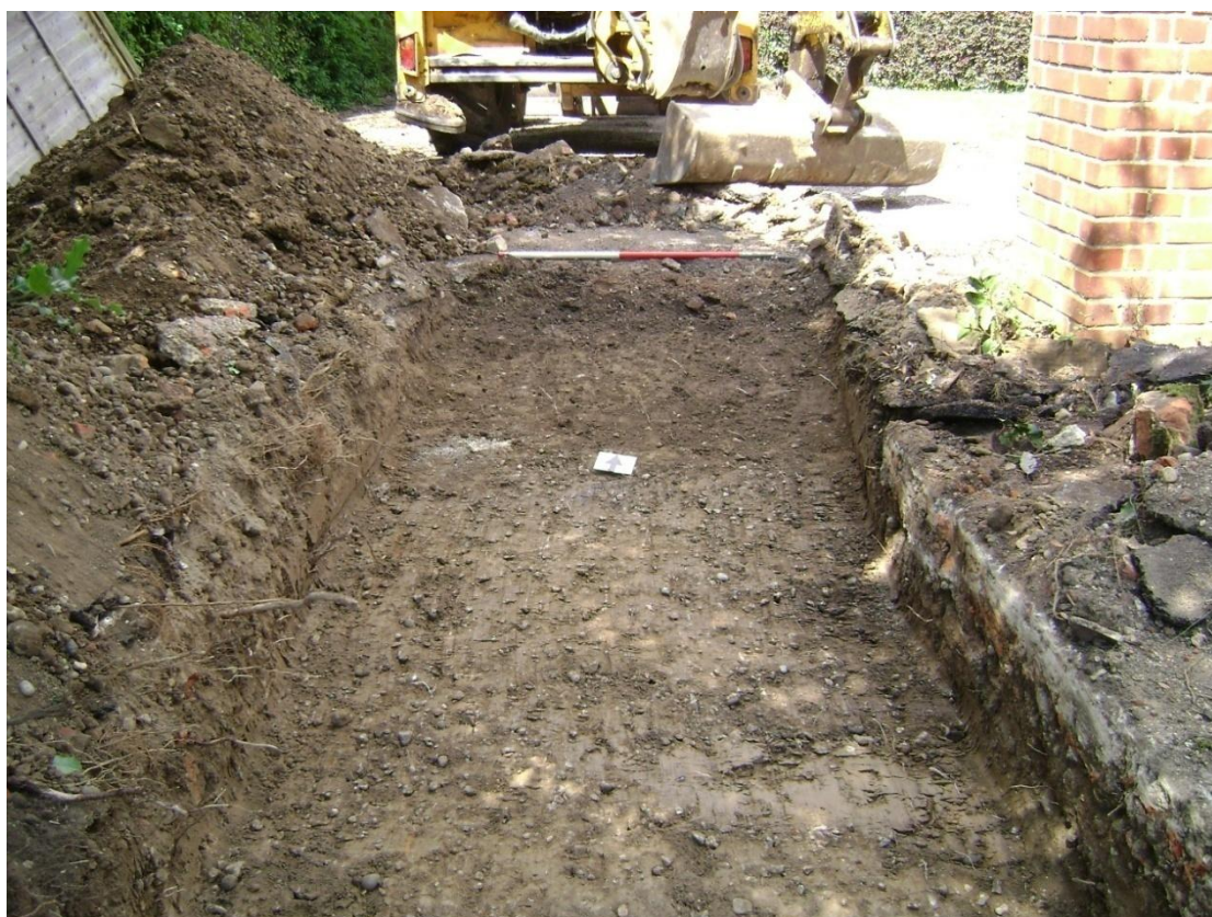
Figure 9. Additional 4 metre extension to north end of trench Looking north-west, 1m scale
