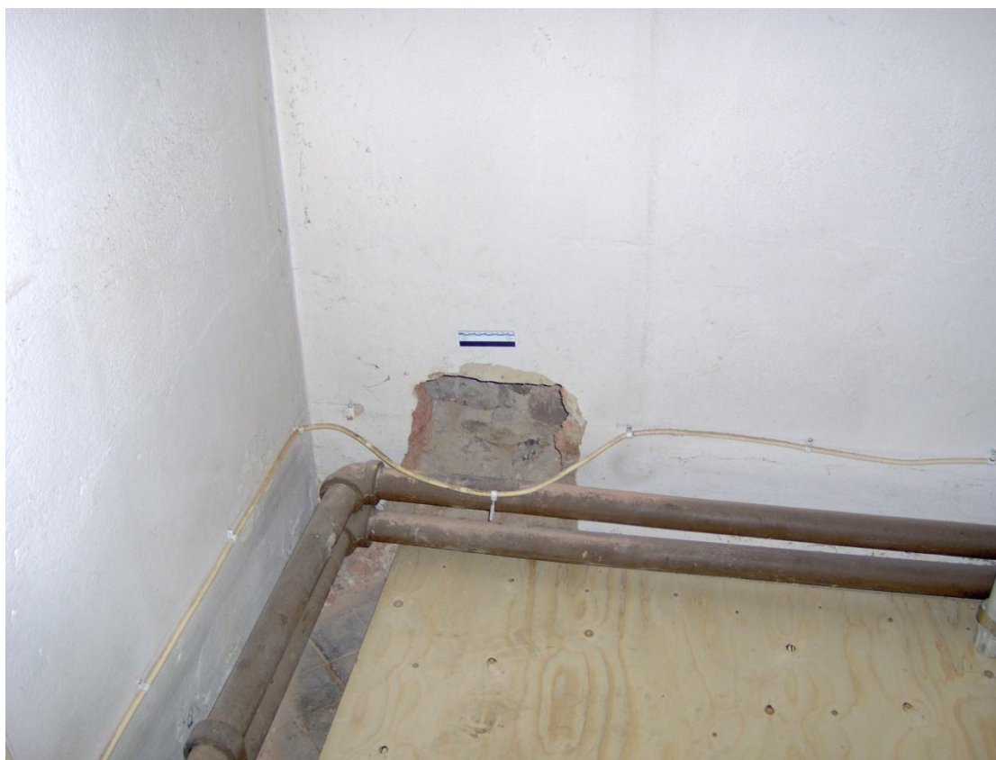
Plate 5: Hole in wall in north aisle showing brickwork with unfaced stone rubble behind, looking north
