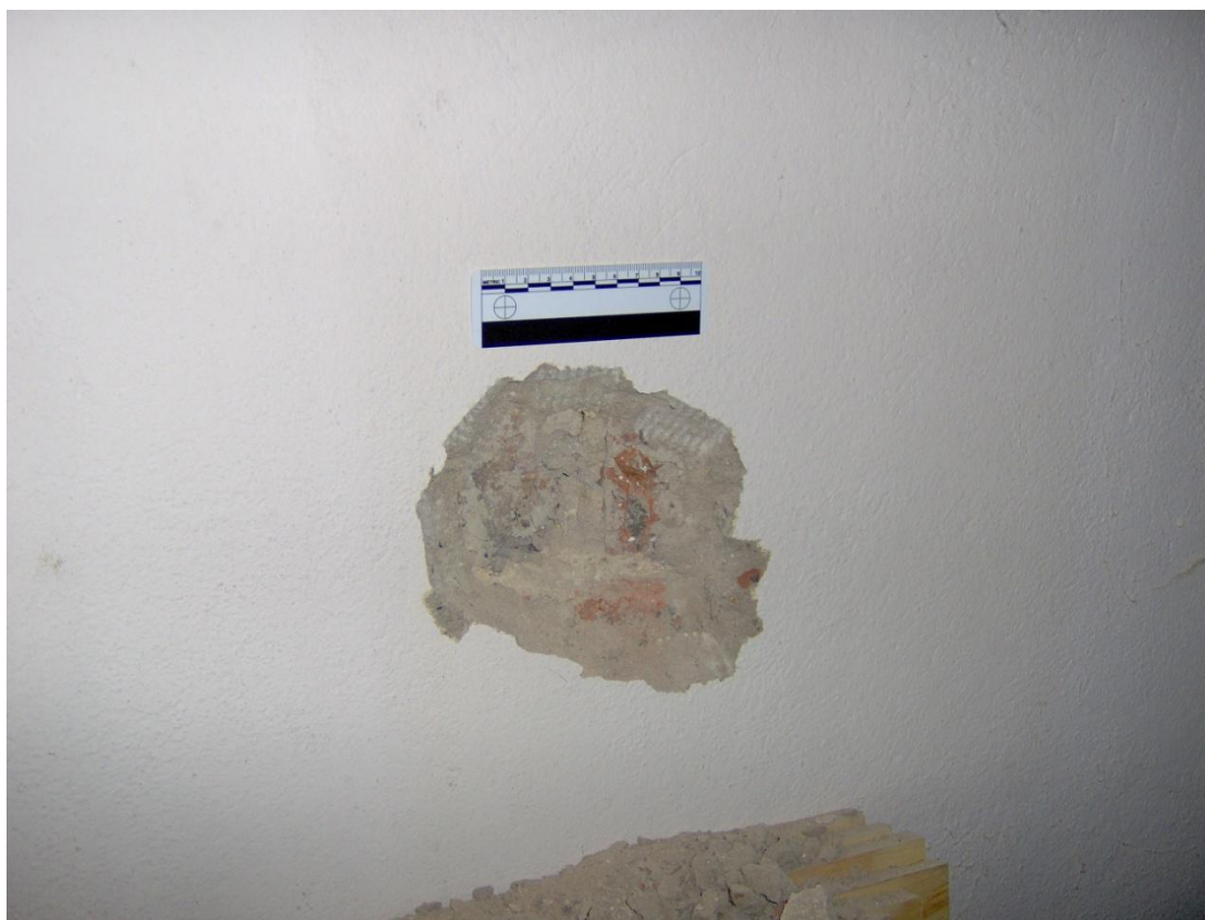
Plate 7: Test slot in north transept showing brickwork behind cement render, looking west
