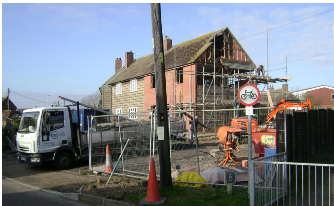
Figure 4 18 Chapel Lane showing that it has had its concrete ship lap skin removed. Looking north-west
