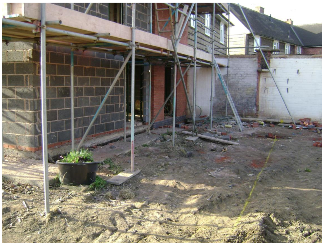
Figure 6 Site before foundation trench excavation looking south. The yellow paint line indicates trench location. The painted white wall is the rear of the adjacent property's toilet block.
