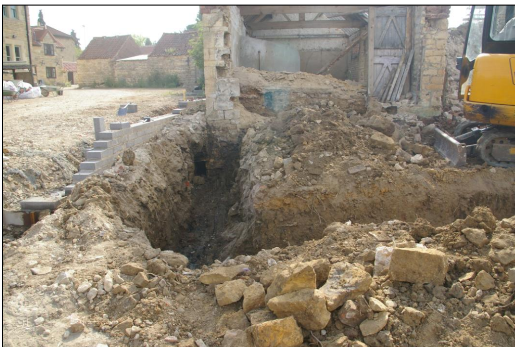
Figure 26. Detail of above, with opening for drain located beneath northern wall of existing building. Looking east.
