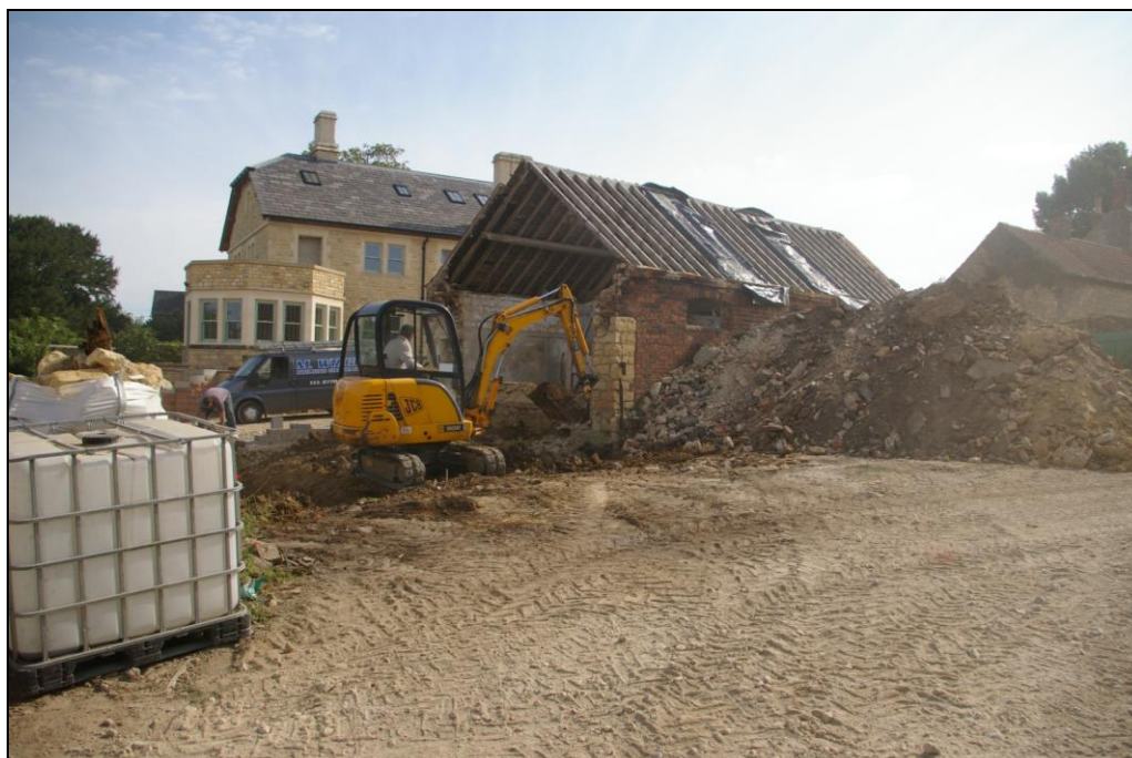
Figure 24. Excavation of footings on the western side of the 19th-century cowshed. Looking north.
