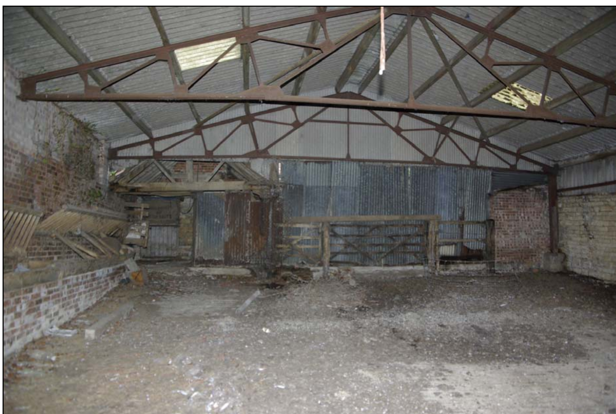
Plate 28. Infill structure interior, with brick feeding troughs and timber hayracks. Looking east.
