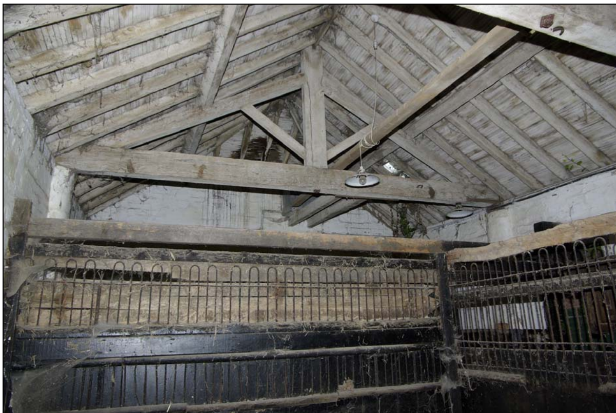
Plate 30. King post roof truss and timber partition walls forming stabling for horses at southern end of cow-shed. Looking south.
