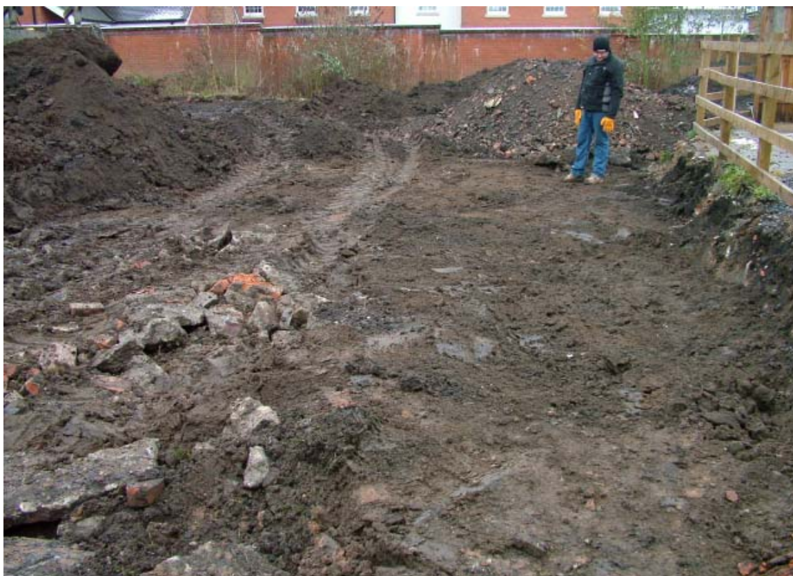
Plate 3: Area stripped of topsoil close to west corner of site, looking east
