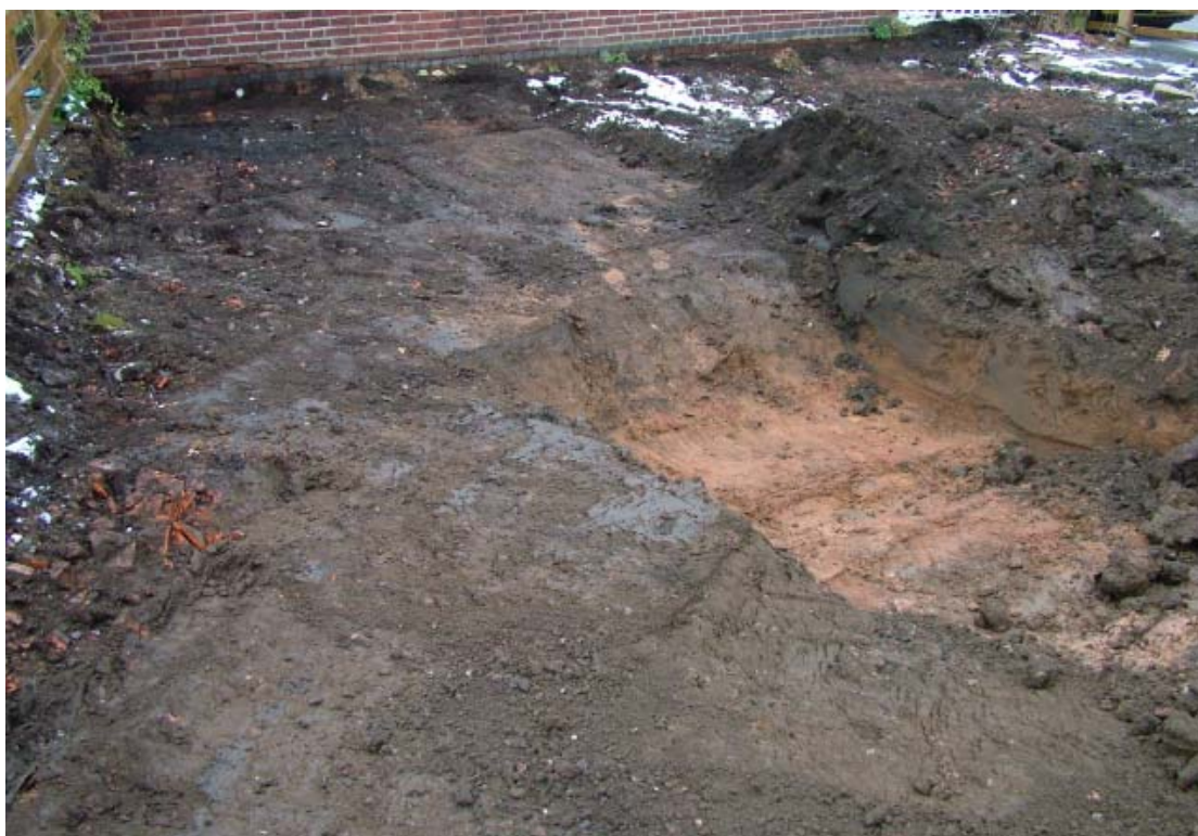
Plate 6: Excavation of waterlogged area to western side of site, showing natural substratum. Disturbed area to left and rear of picture
