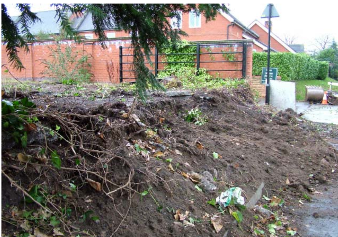
Plate 2: Proposed entranceway prior to excavation and after removal of railings and shrubs, looking east northeast
