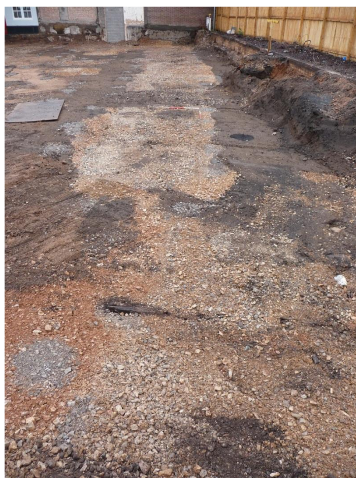
Figure 18: Southern area following machining to formation level with western edge of site to right. View looking south; 1m scales
