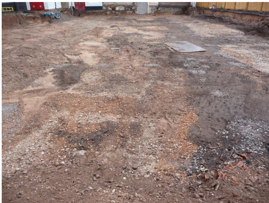
Figure 17: Southern area following machining to formation level. View looking south; 1m scales
