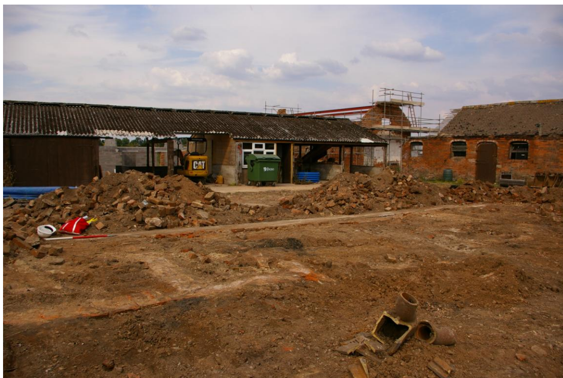
Plate 11: The beam and brick foundations to south of central range, looking north-east
