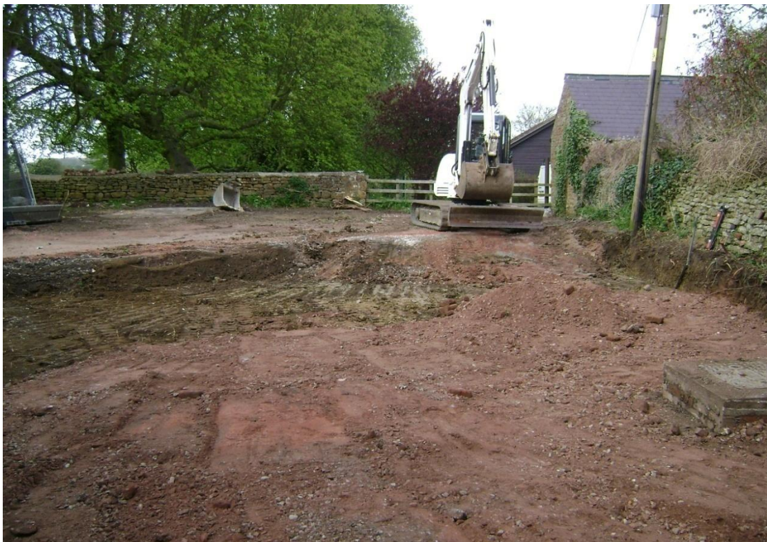
Figure 5. After site reduction. The concrete garage bases remain to be removed in the north end of the site. The raised cover of the sewer pipe can be seen on the right of the picture. Looking north
