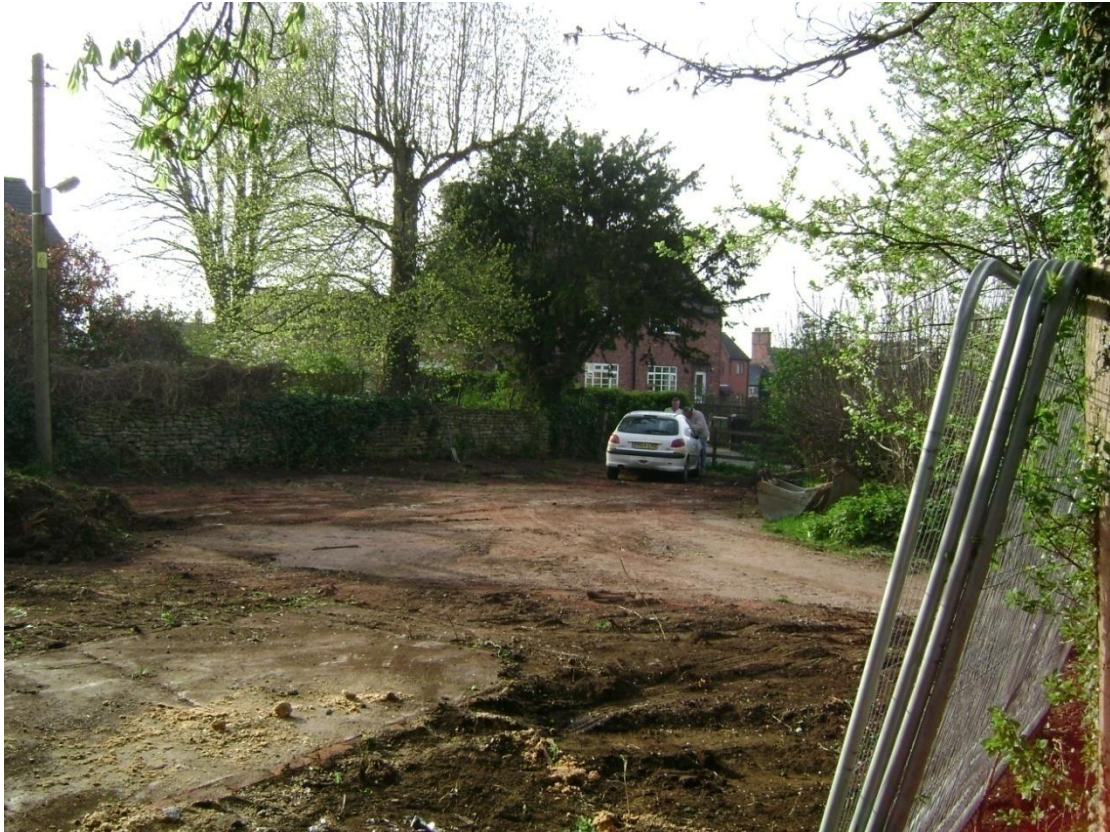
Figure 4. Site after removal of vegetation and before level reduction Location of garage base can be seen in foreground on left of picture. Looking SE
