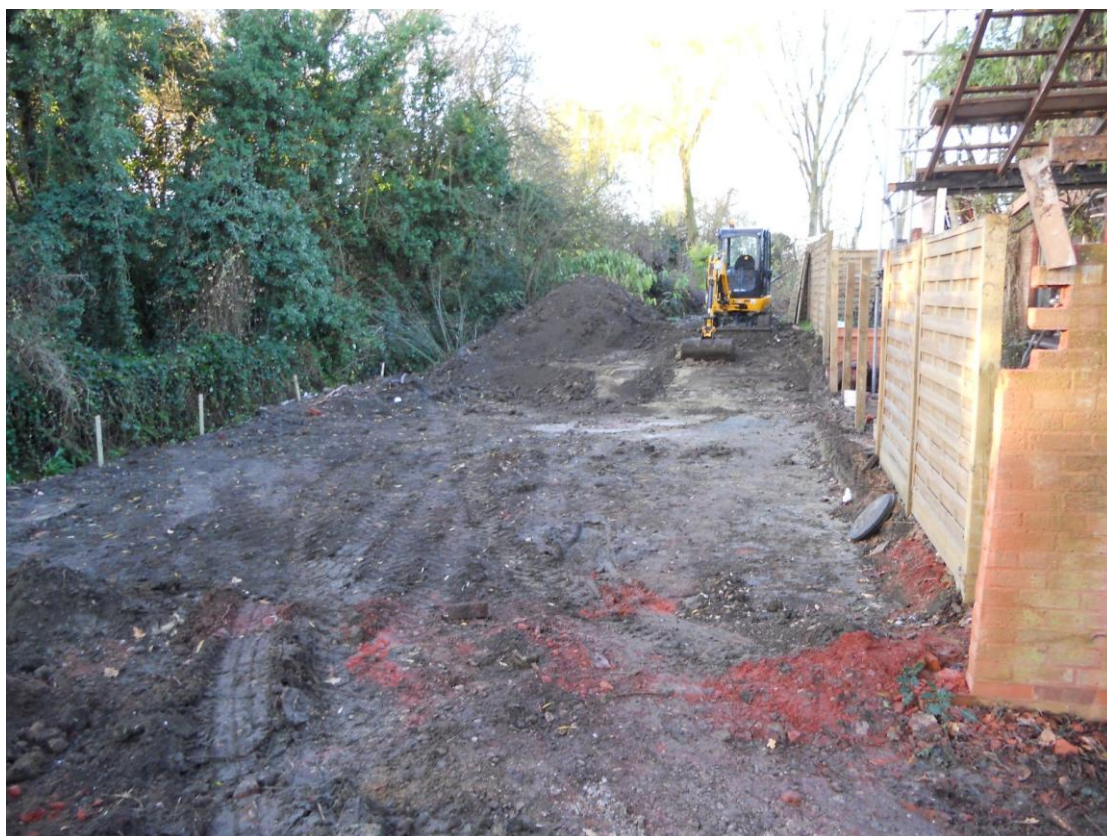
Figure 5. Levelled site Looking west. Note exposed natural at far end of terrace near excavator
