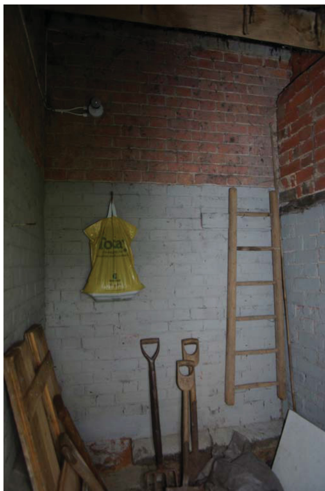
Figure 12. Interior of store, looking south onto north-facing wall of tower, site of proposed entrance to new extension.
