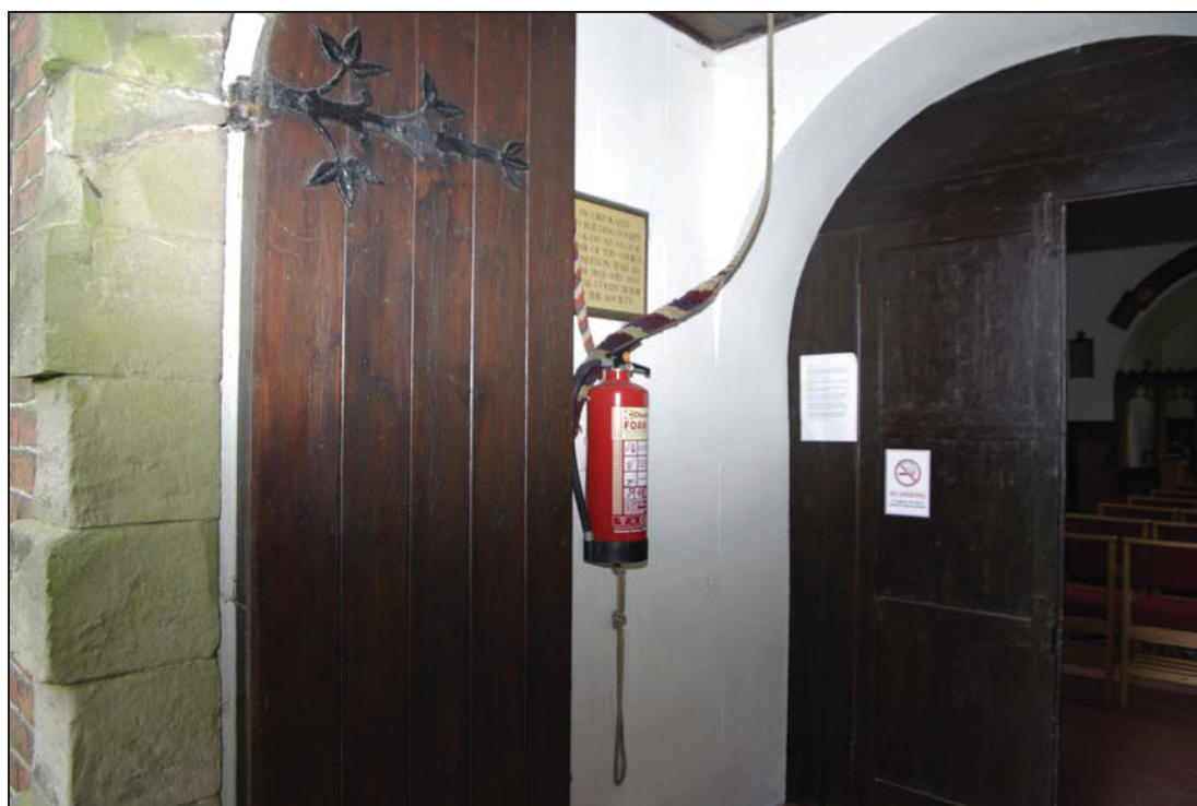
Figure 9. Porch entrance at base of tower: site of proposed doorway into new extension. Looking north-east.
