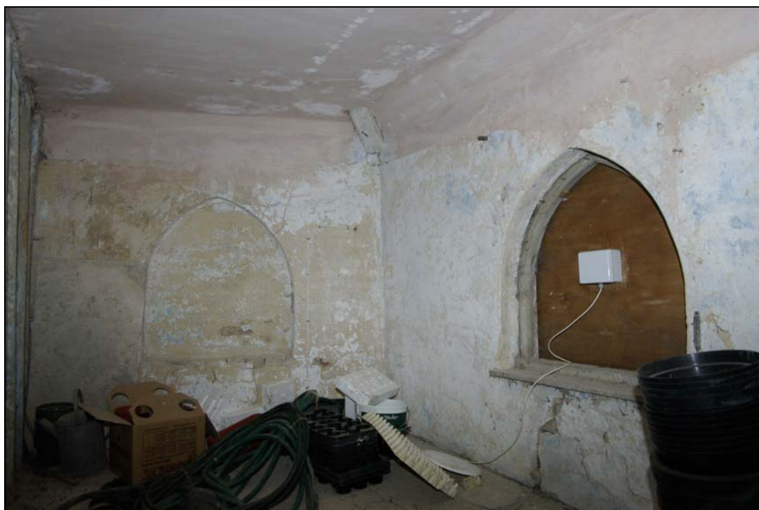
Figure 14. Boarded upper floor window light. Looking south-west.
