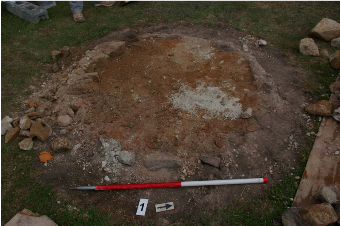
Figure 7. Pier 1, following dismantling, showing mortared granite wall and loose infill. Looking west.
