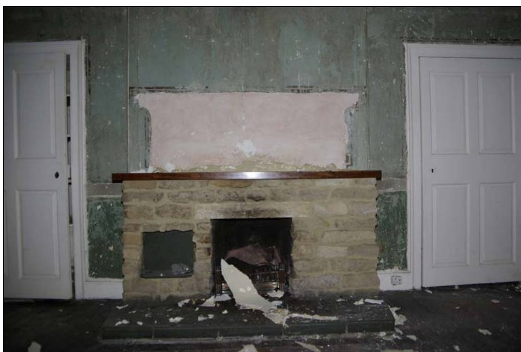
Plate 14. Ground floor reception room, with outline of 18th fireplace visible in plasterwork behind modern replacement. Looking east.
