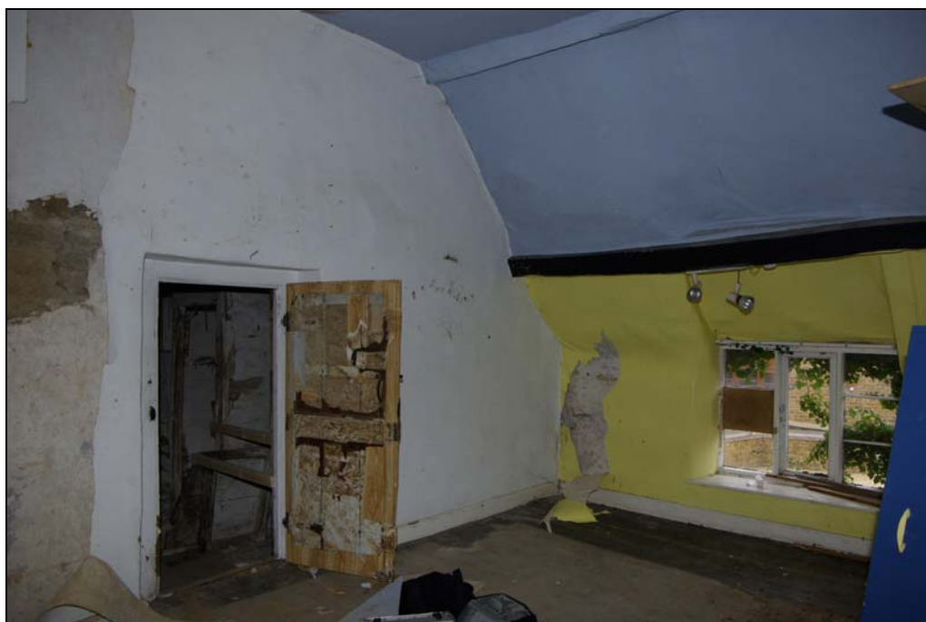
Plate 19. First floor chamber, with two tiers of side purlins visible. Looking south-west.
