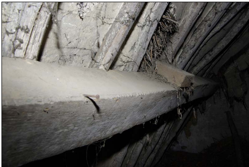
Plate 27. Detail of notched side-purlin, supporting modern timber, part of the external framework which supports the 20th century tin roof cover. Looking east.
