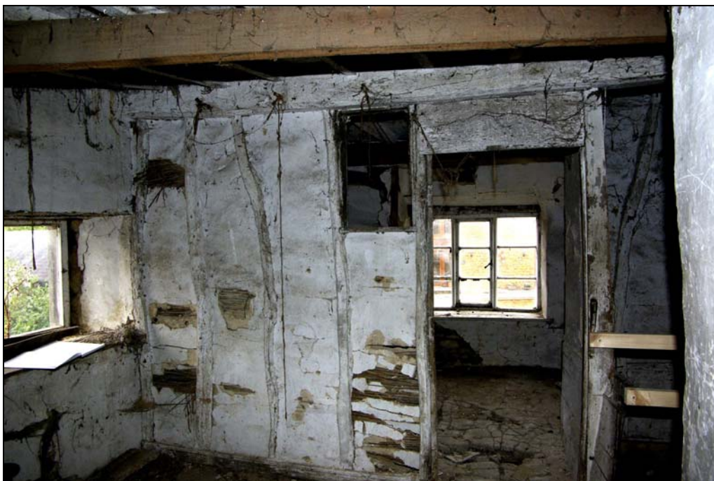
Plate 22. Southern service end bay, first floor, with early stud partition wall. Looking west.
