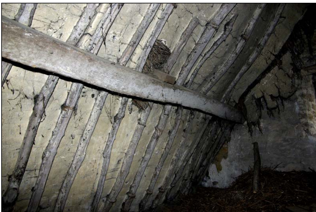
Plate 26. Detail of roof structure, showing ash-pole rafters with twine ties securing thatch bundles. Looking east.
