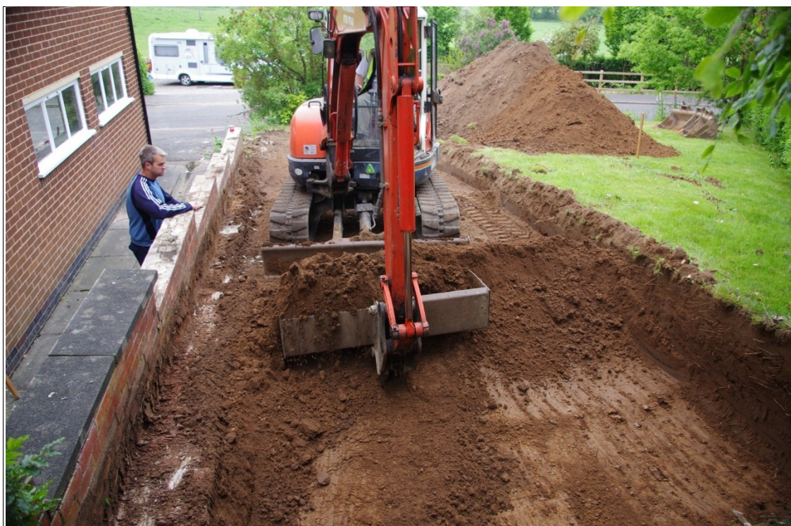
Figure 3 Stripping the area north west of the present house. Looking south west
