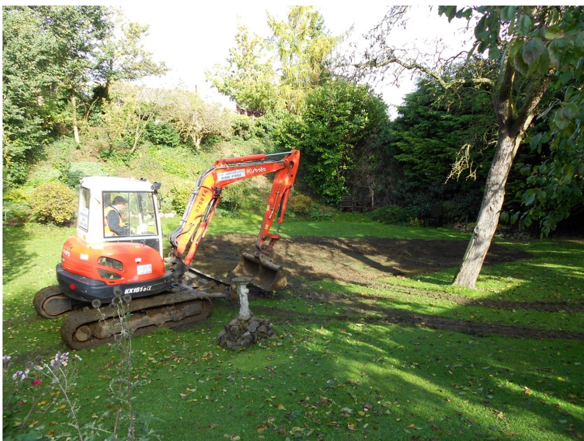
Figure 5: Backfilled Trench 2, and to the rear the large bank, seen on early OS maps
