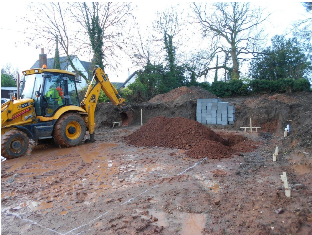
Figure 4: Site view showing the depth of reduced ground along the northern and western edges of site. Looking west.
