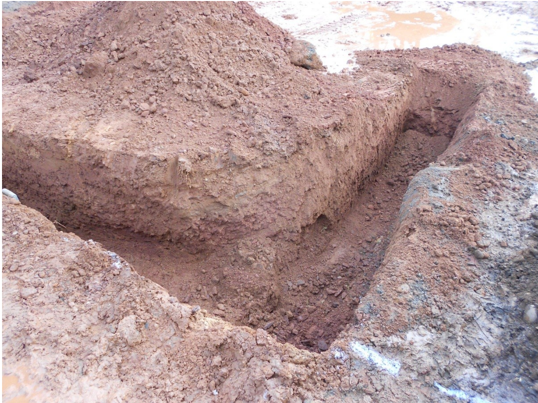
Figure 5: View of south-west corner of foundation trench, showing natural sand and gravel. Looking north-east.
