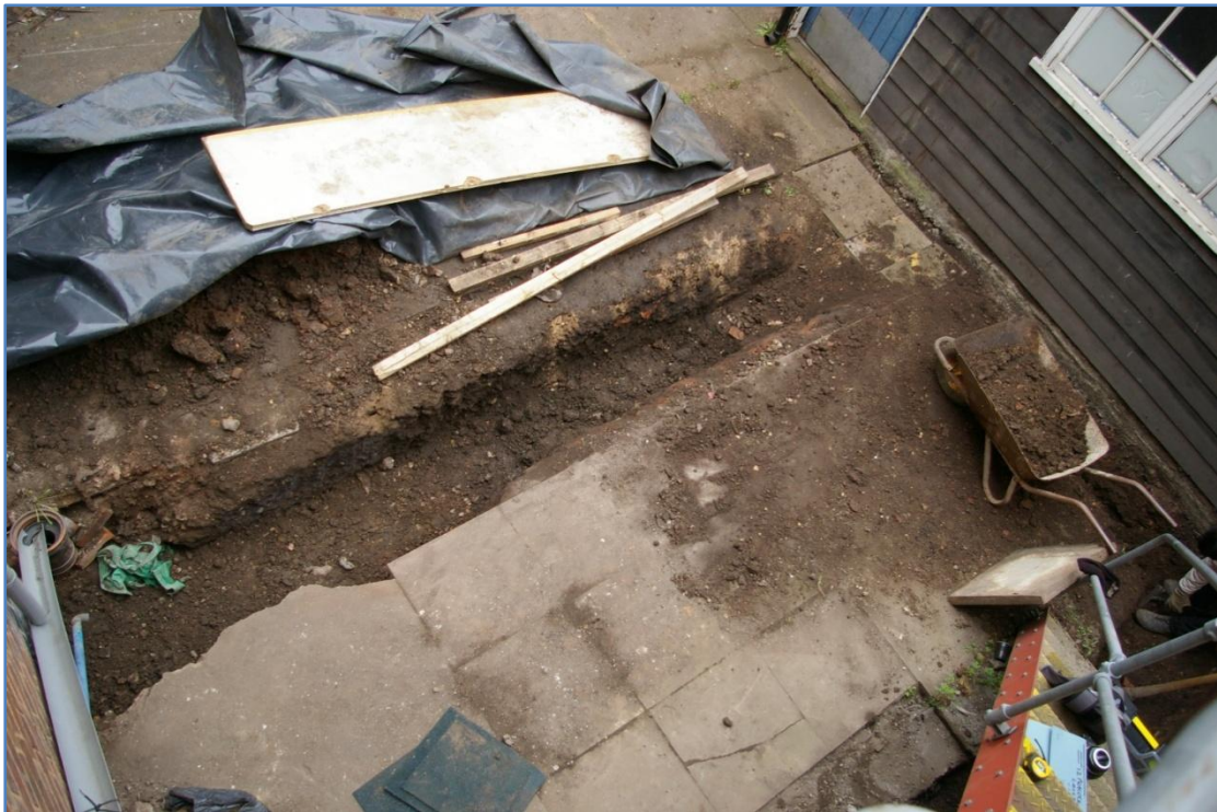
Figure 3 The east trench in the course of excavation. From above, looking south-east.
