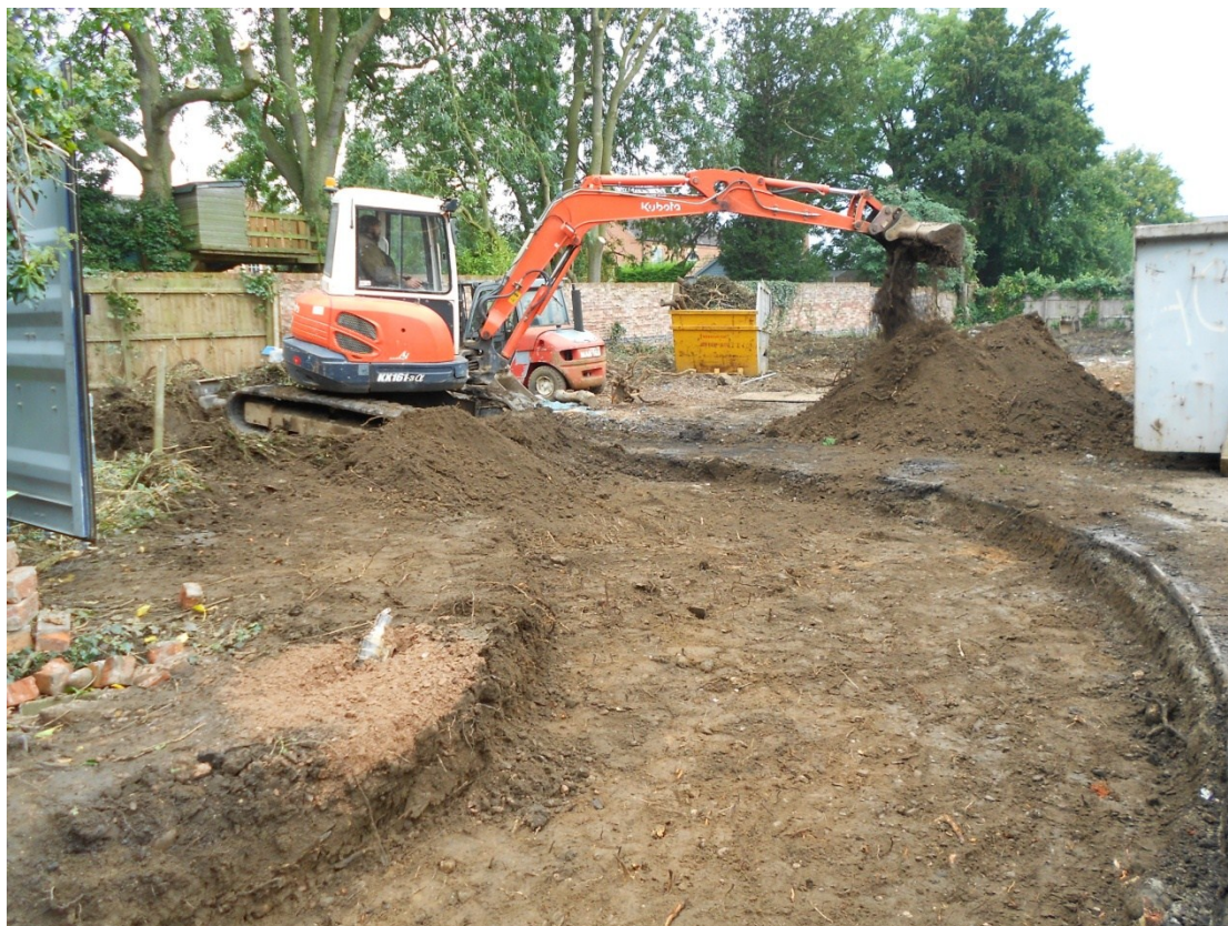
Figure 3: Machine removal of garden soil in area of access road; view northwest
