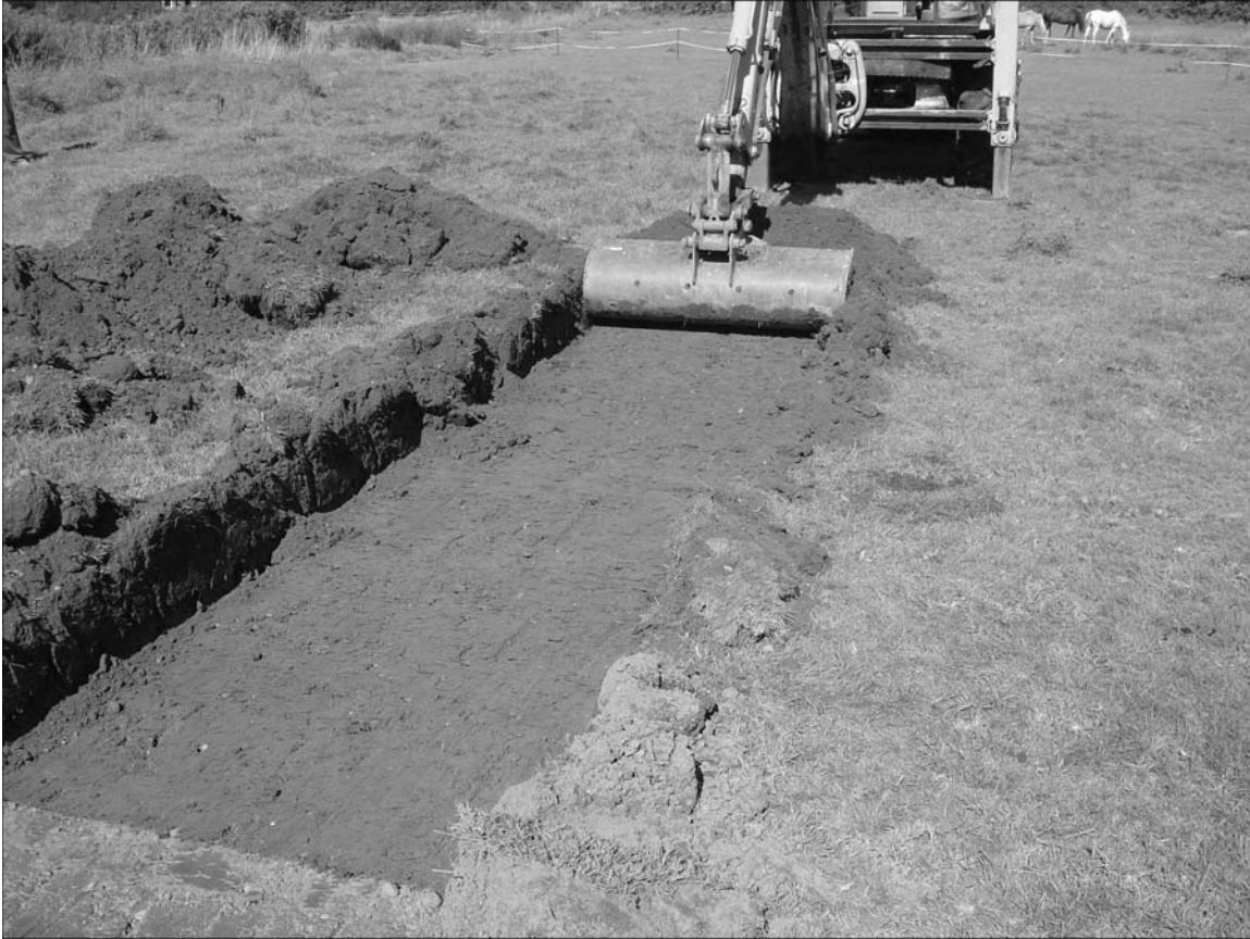
Fig. 4. Photograph of topsoil and subsoil stripping in area of stable block and hard standing, facing north.
