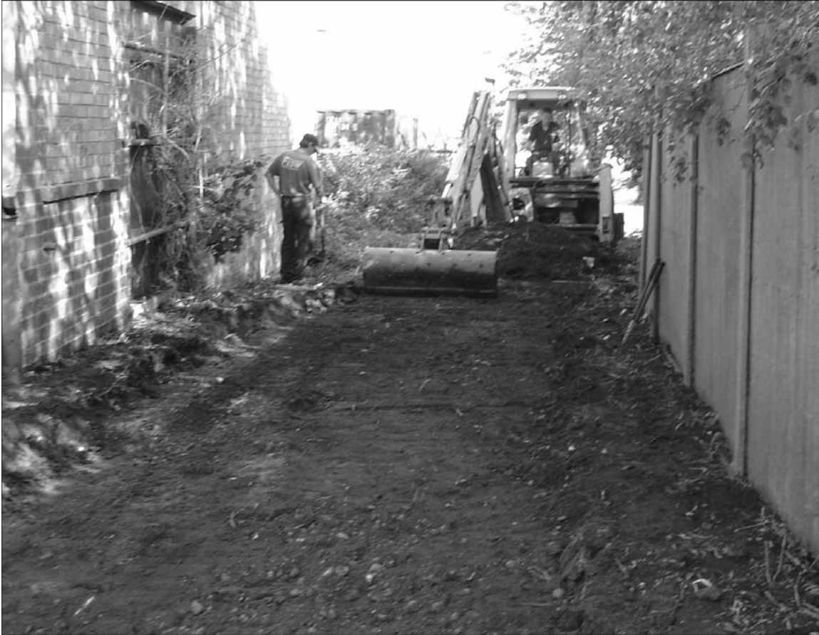
Fig. 3. Photograph of topsoil stripping in the area of the driveway, facing north.
