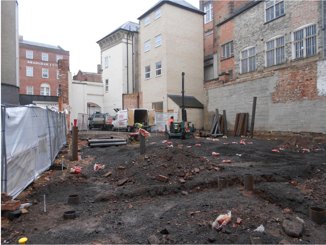
Figure 3: General view of the site looking south-east, showing finished ground-beam trenches in the foreground.
