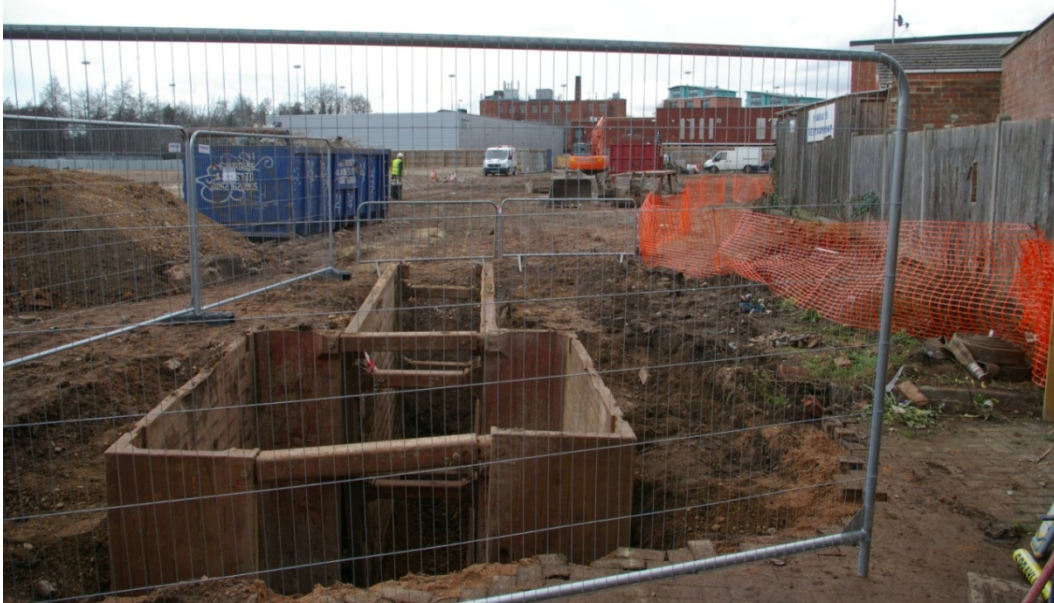
Fig. 4: Box prop support in service trench adjacent to Foxon Street (looking north)...
