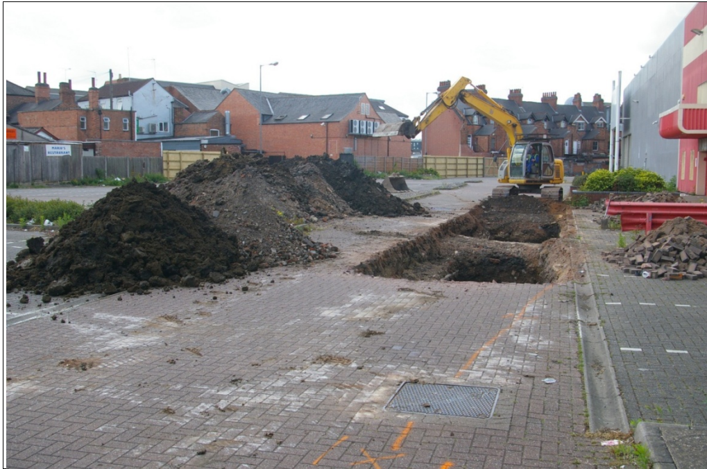
Fig 5. Machining Trench 4 within the footprint of the proposed building, and to the east of the current buildings. Steps left in for live services. The proposed building extends beyond the spoilheaps and to the edge of the red building (Carpet Right). The 1970s excavations took place to the left and towards the fencing.
