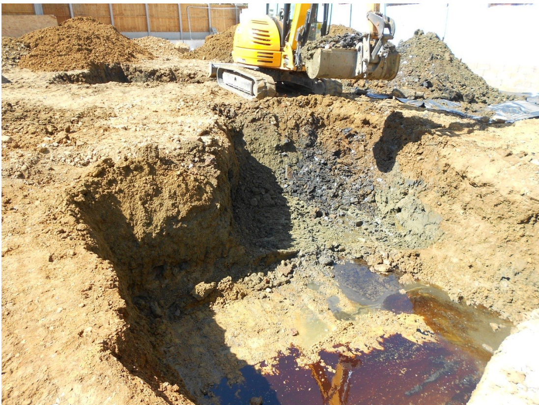
Figure 6: Pit containing oil-contaminated glass (beneath digger bucket), looking north-west from Church Lane frontage.
