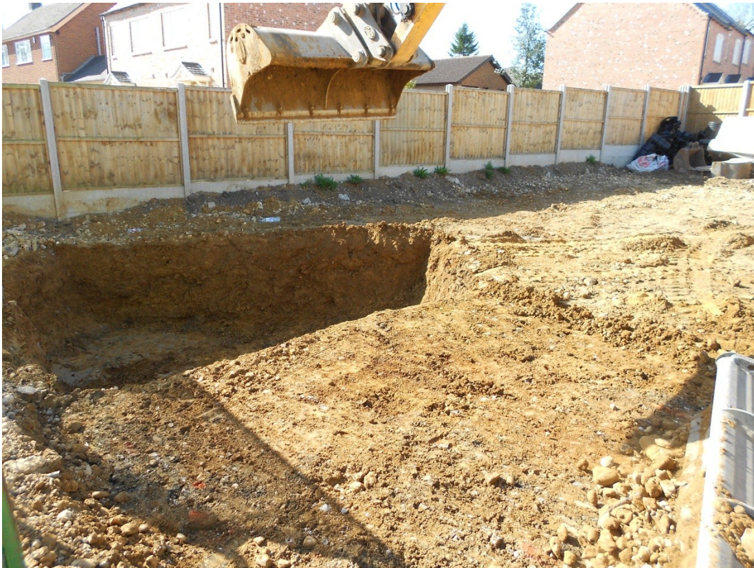
Figure 4: Typical area of natural ground with overburden removed in site's south-east corner. Looking south.
