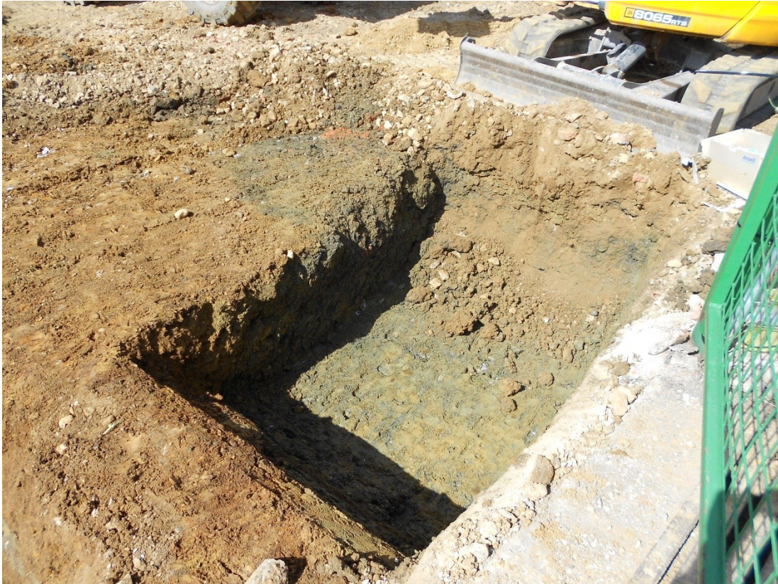
Figure 5: Discolouration of ground from diesel contamination on Church Lane frontage. Looking north-west.
