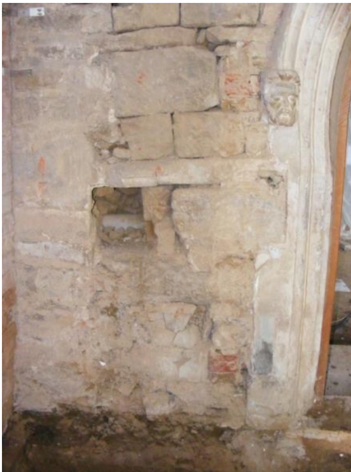
Figure 7: The exterior of the north aisle wall, as seen from inside the north porch (trench M below)
