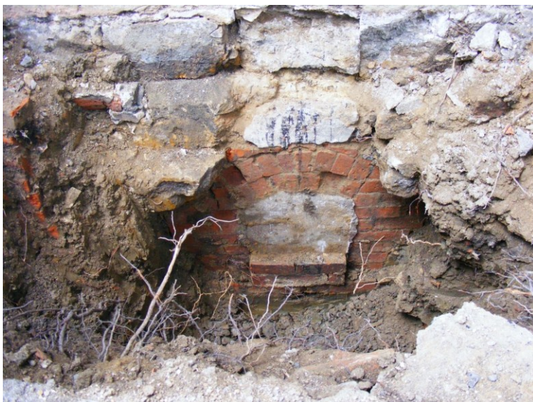
Figure 6: A possible vent for the heating system, as seen from the exterior following removal of the brick shaft
