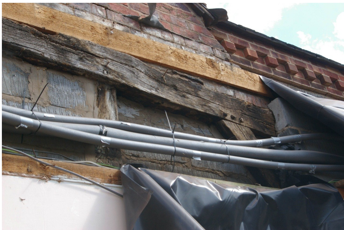
Plate 5: Part of box frame of original house, exposed after demolition. Looking north-east
