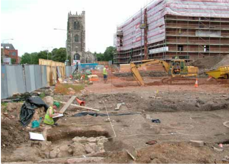
Fig. 9 Sanvey Gate frontage area excavations, and machine excavation of the town ditch sections ongoing. Looking east.
