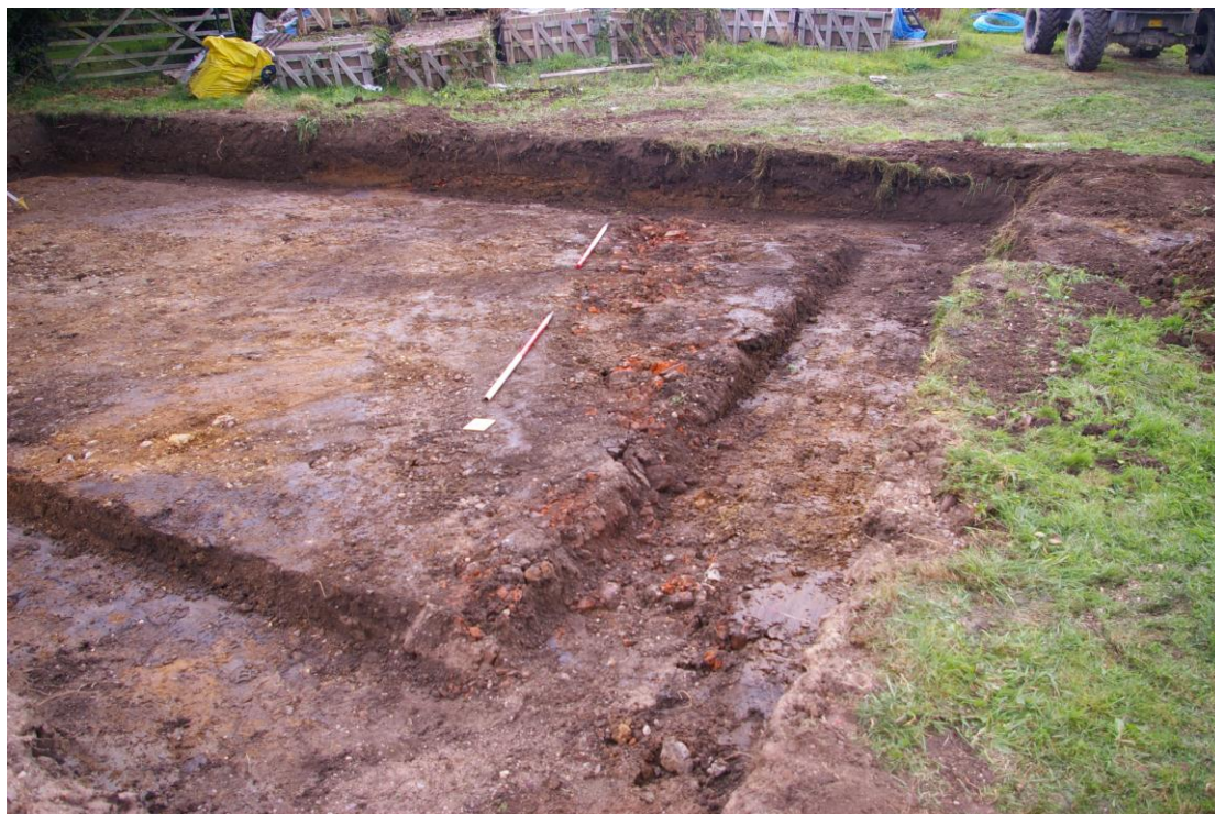
Plate 9: Demolished wall and rubble at southern end of footprint, looking east north-east
