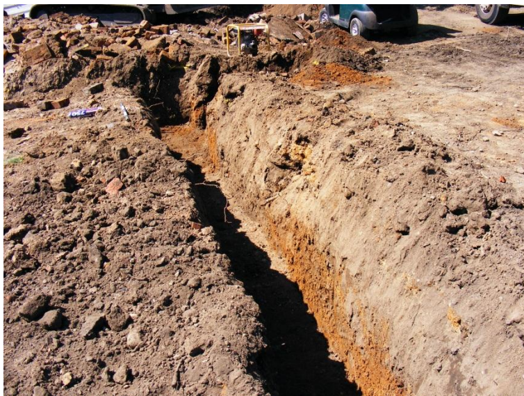
Figure 7: Footing trench running NW-SE in the centre of the house footprint. Disturbed ground can be seen in the centre of the trench.
