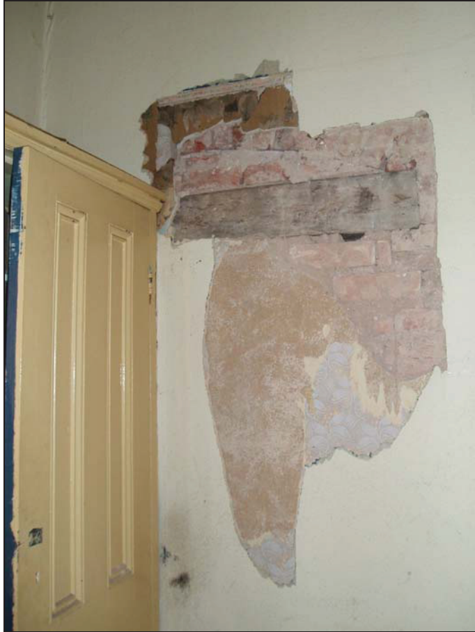
Plate 7. First floor landing, showing C19th cupboard and blocked doorway through to 59a Highcross Street. Looking north.
