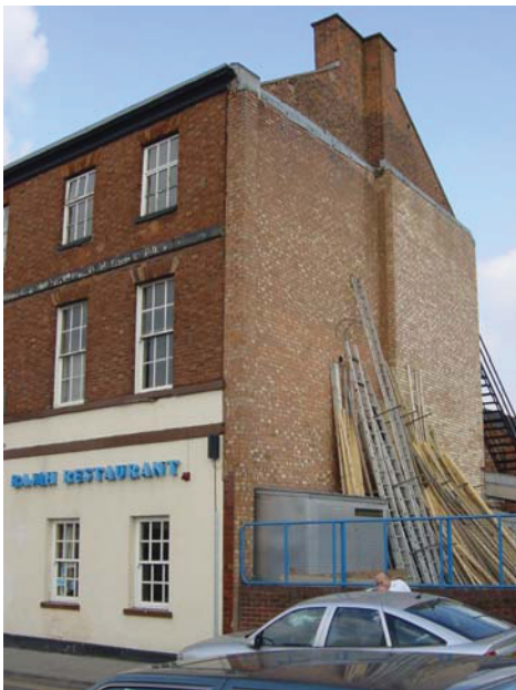
Figure 1: Grade II listed No.59 Highcross Street. Note the 'skin' wall against the southern gable end.
