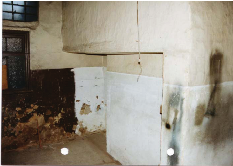
Plate 16. Room 12. Rear of large chimney stack, taken prior to 1990s redevelopment. Looking south-east. Photograph supplied by N. Weafer.
