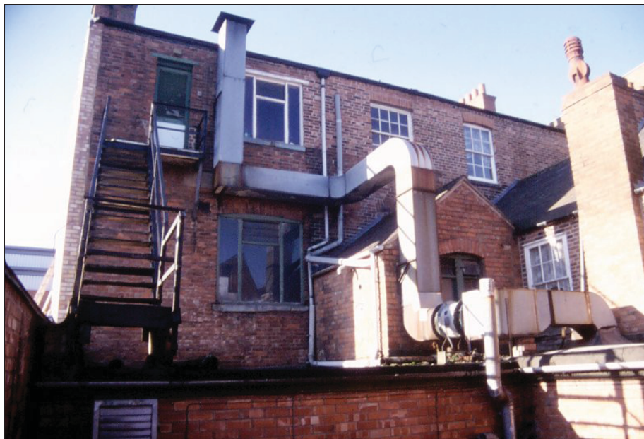
Figure 1. Rear of 59 Highcross Street showing the first floor section of the 19th century two-storey range (behind extractor ducting).
