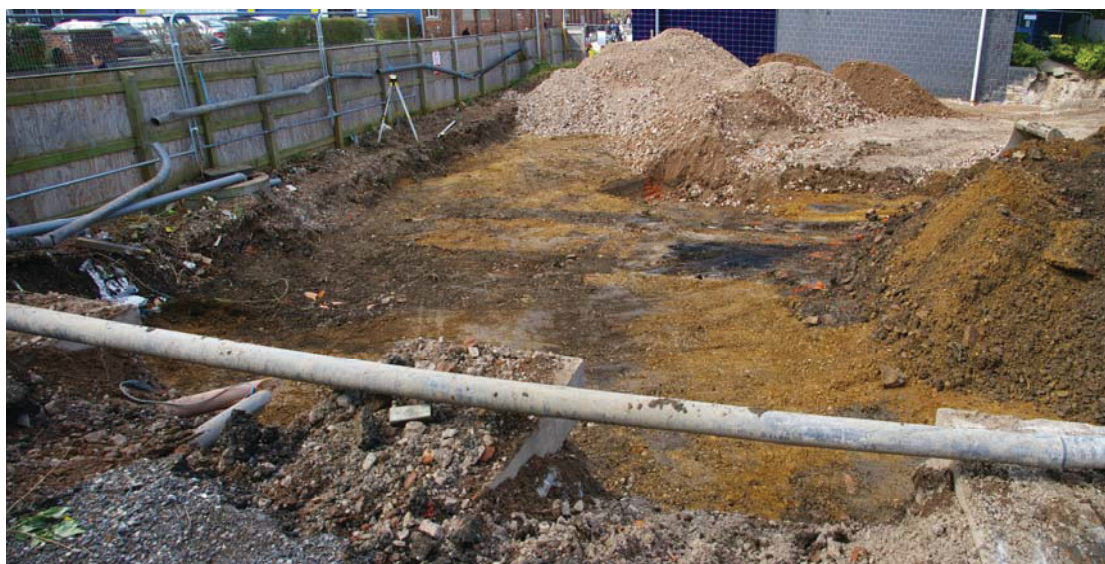
Plate 13: The western part of the site from the south, showing services and concrete stanchions
