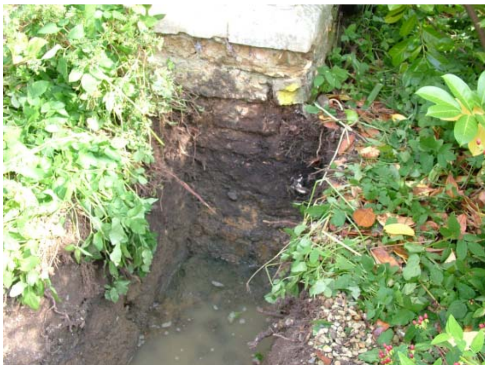
Plate 5: North west facing elevation of house foundations (southern side), looking south east
