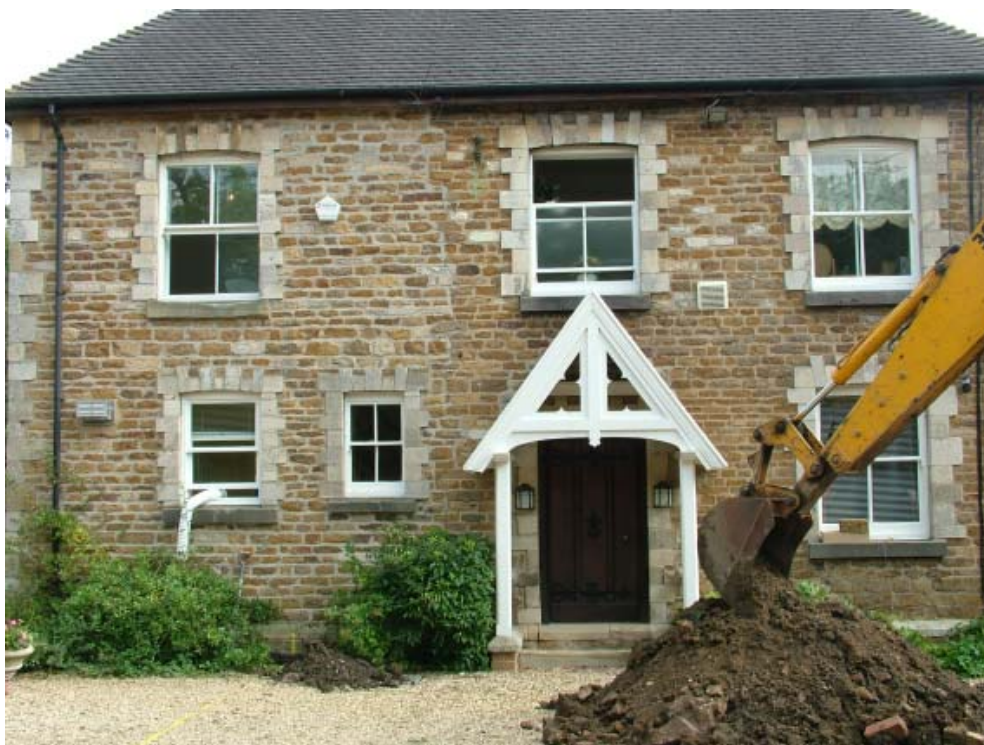
Plate 1: North west facing elevation of Woodend Cottage, showing differential builds, looking east
