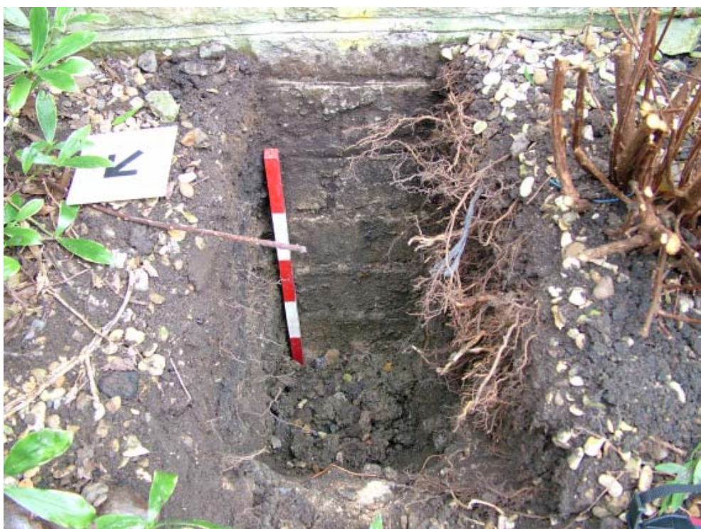
Plate 4: North west facing elevation of house foundations (northern side), looking south east
