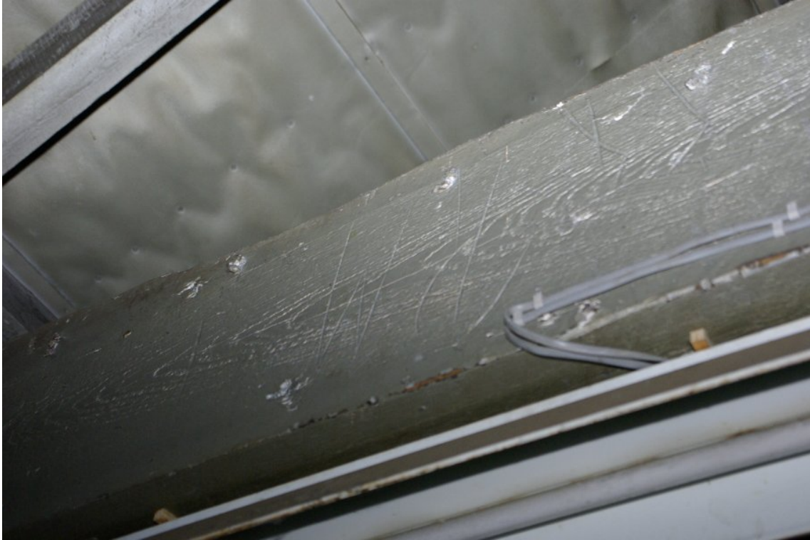
Figure 24 Inverted RM on tie beam, building 4.
