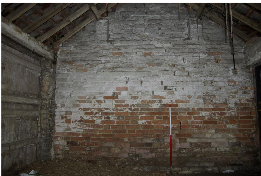
Figure 16. West building, east gable wall Looking east at the different sizes of bricks used. 1m scale
