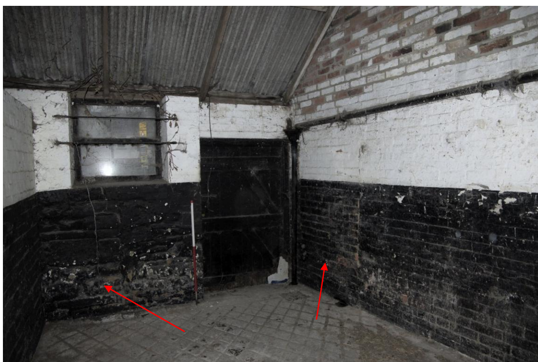
Figure 9. East building, eastern room Looking north-east. 1m scale. Note blocked doorways in north-eastern and north-western corners marked with arrows
