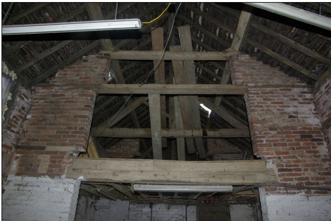
Figure 12. Inserted brick piers in Barn, with king-post roof truss behind. Looking east.
