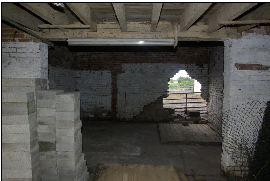
Figure 13. Western gable-end wall of Barn, with doorway broken though into stockyard. Looking west.
