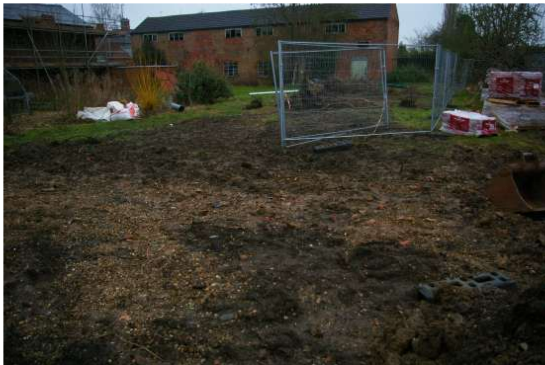
Figure 6 Location of drive before excavation Looking north east. Building 1 on left of picture, Building 2 in centre
