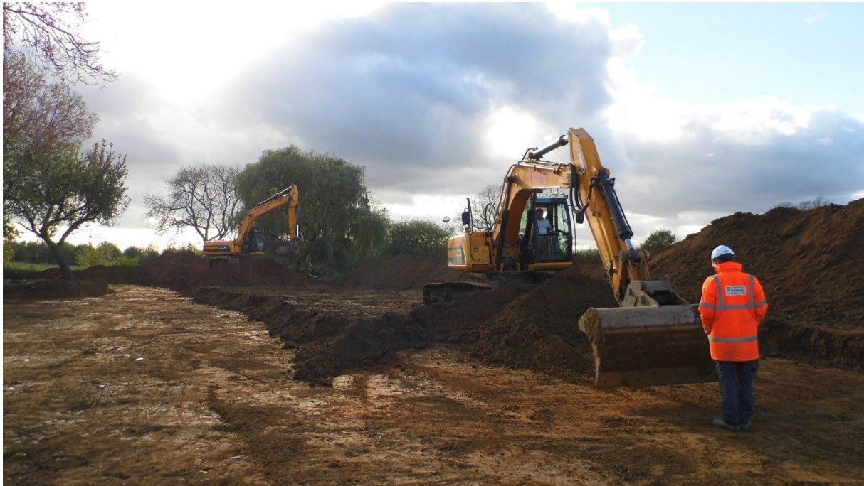
Figure 4: Area 1 – supervising overburden removal at the eastern end of Area 1, looking south-west
