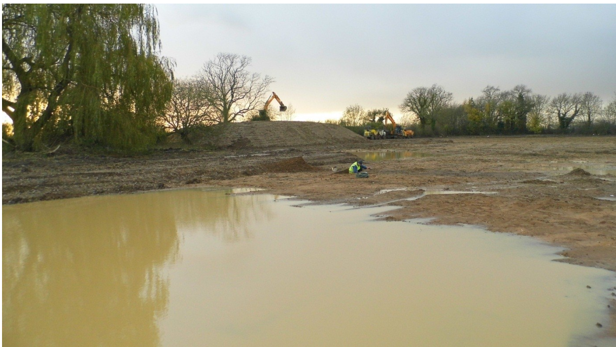
Figure 5: Area 1 - flooding during the excavation meant that large areas of the site were unexcavatable.
