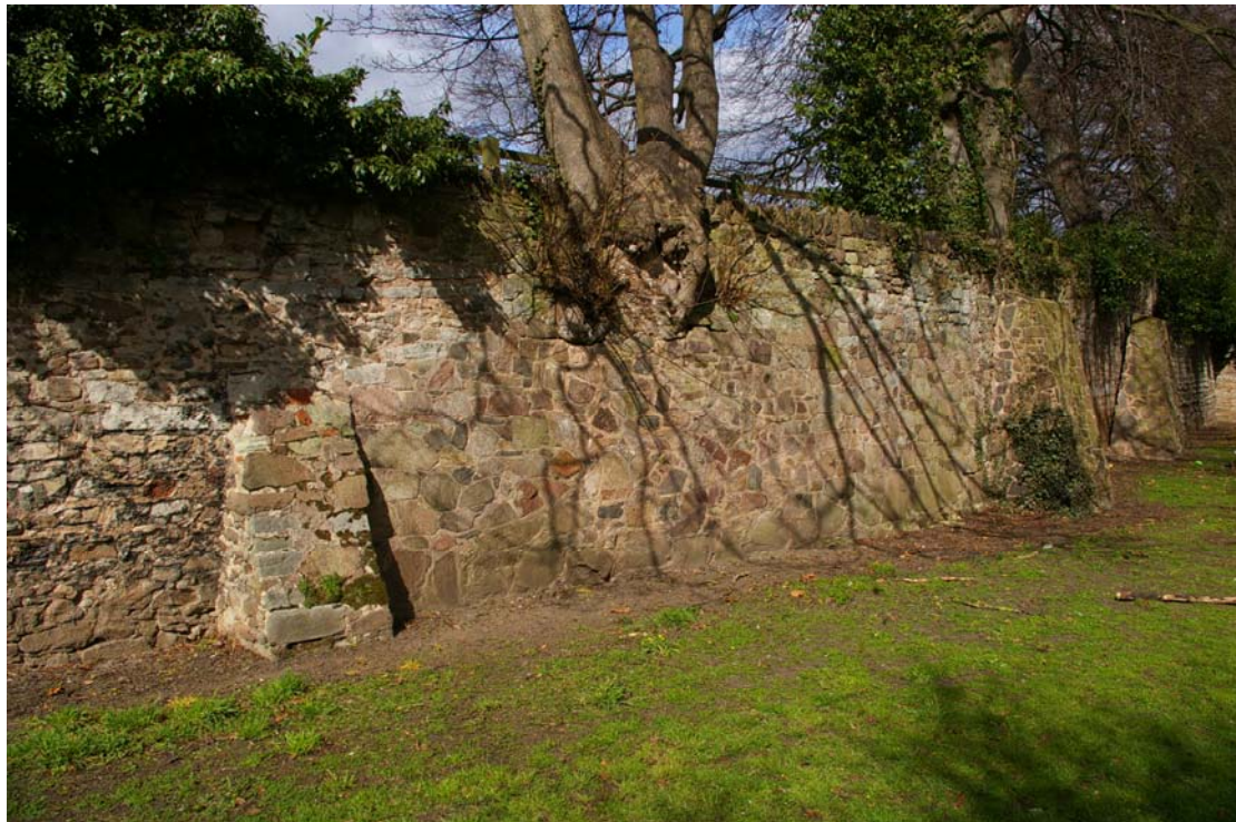
Figure 3 Eastern face of precinct wall Looking north west. Trench and boreholes on opposite side of wall
