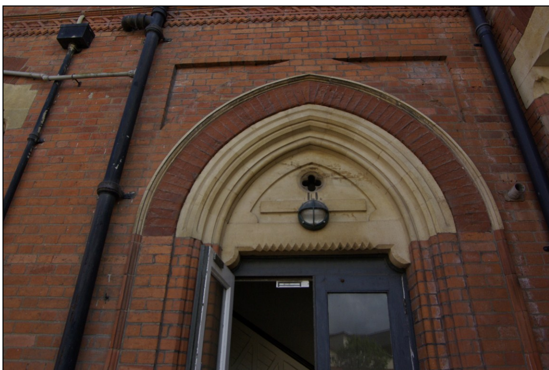
Figure 24. Former entrance to boys' school, showing decorative detail to arch-headed doorway opening, with roll moulding and nail head motif. Looking south.
