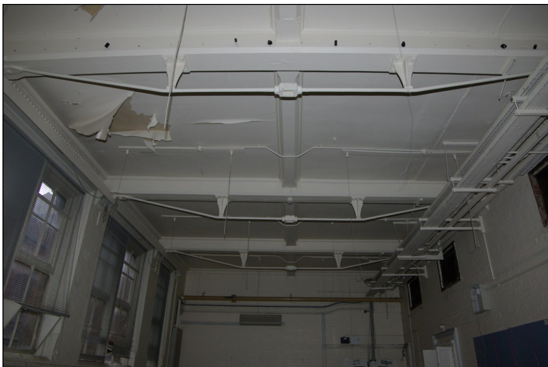
Figure 30. Former mixed school room, with chamfered and stopped timber axial and transverse ceiling beams. Looking west.
