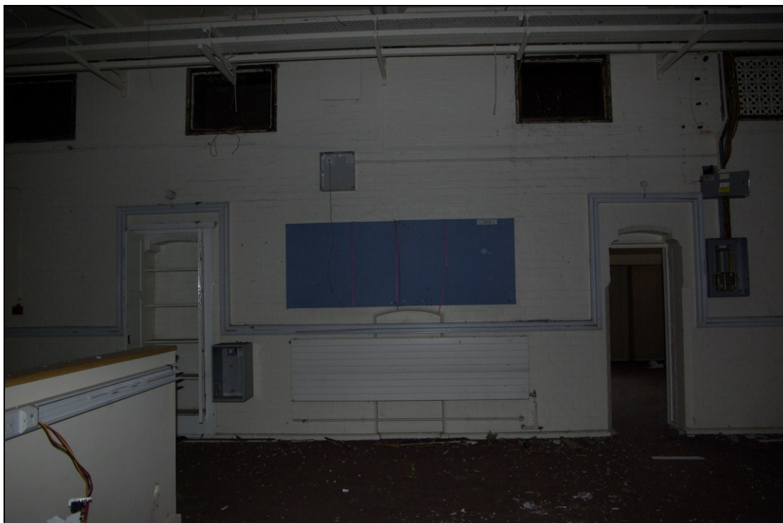
Figure 31. Former mixed school room, showing shouldered-arch doorway openings (converted as a cupboard on left hand side), and blocked fire-place opening. Looking north.
