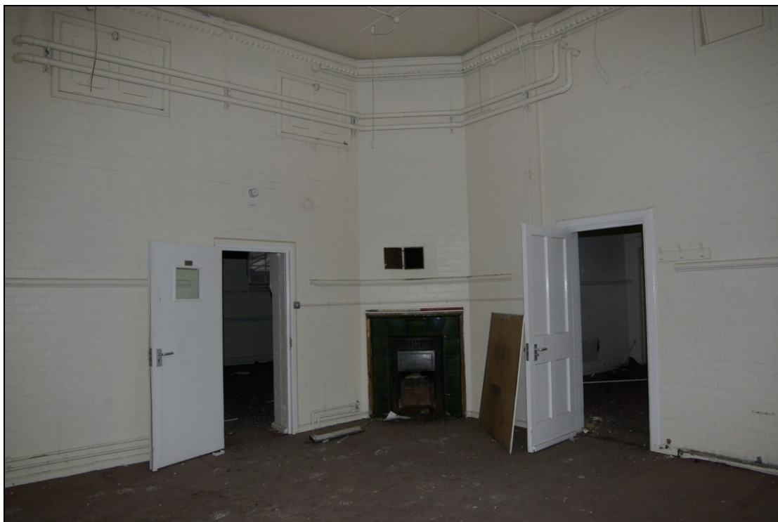
Figure 29. Former heated classroom of 1873, showing decorative brickwork cornice with nail-head motif. Looking south.
