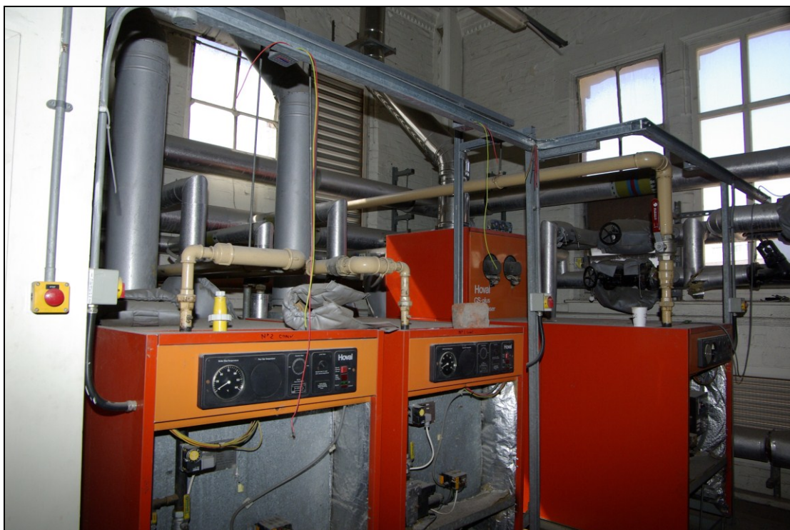
Figure 38. Modern boiler equipment within former class-room, looking west.
