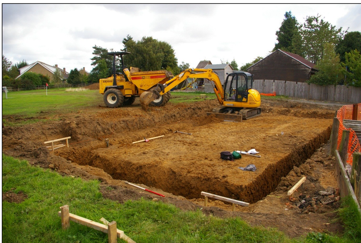
Figure 11. A above, with possible pit (5) [6] on right hand side, against foundation trench. Looking east.
