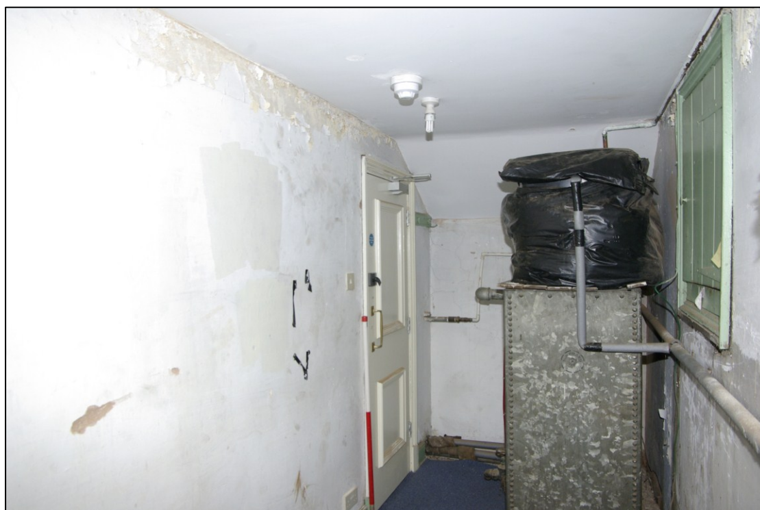
Figure 40. Room S1 Looking north-east. 1m scale. Hatch to roof space on right.
