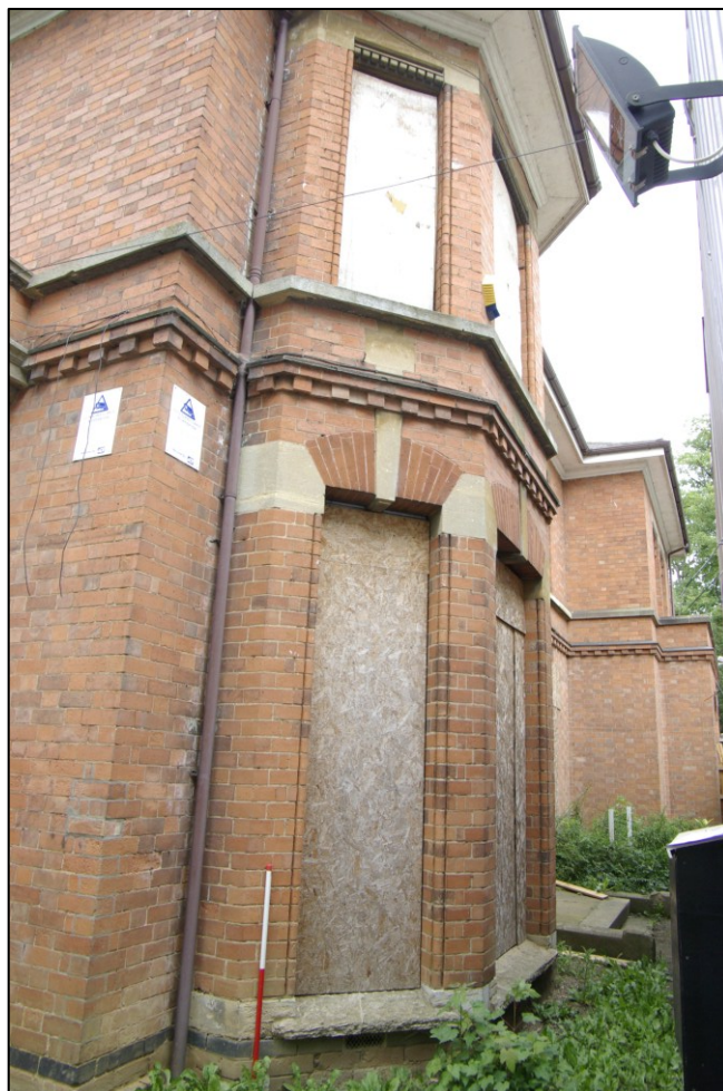
Figure 7. East-facing elevation bay window Looking north-west. Note northern element of façade on right of picture. 1m scale
