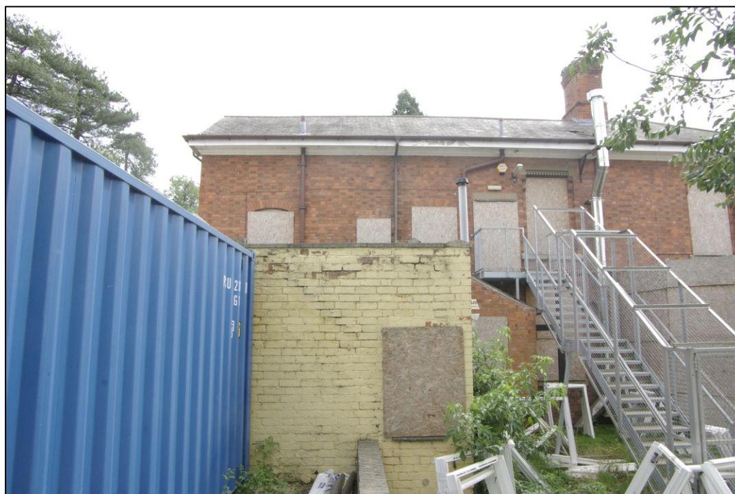
Figure 12. West facing elevation, service wing Looking east. Yellow wall is the rear of the privies
