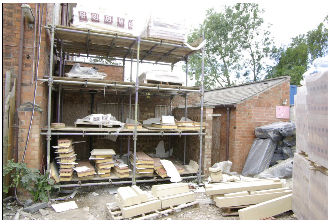
Figure 17. North facing elevation of toilet block. Looking south-west. Note mid-20th century brickwork behind scaffold shelving.
