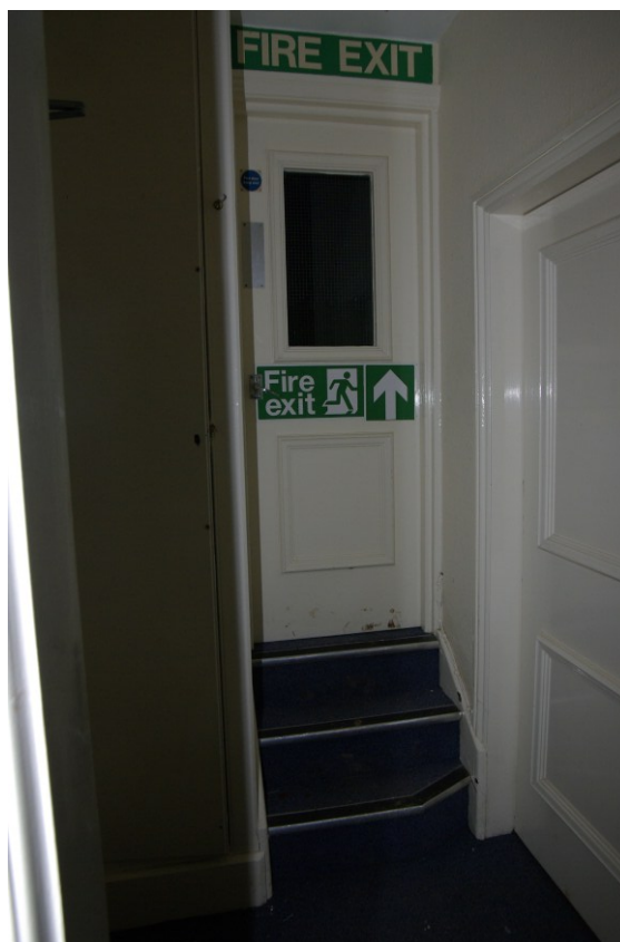
Figure 37 Room F6 and F7 steps Looking south-west. Room F6 at top of steps, Room F7 on right of picture
