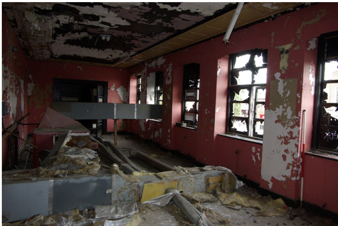
Figure 21. First floor landing Looking north-east. 1.5m scale. Note art deco style ceiling decoration
