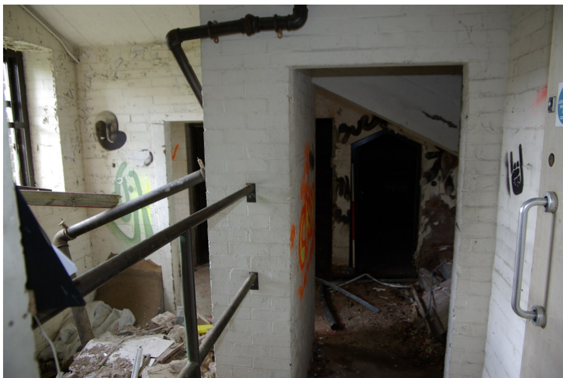
Figure 16. Removed public staircase to south of entrance foyer Looking south. 1.5m scale
