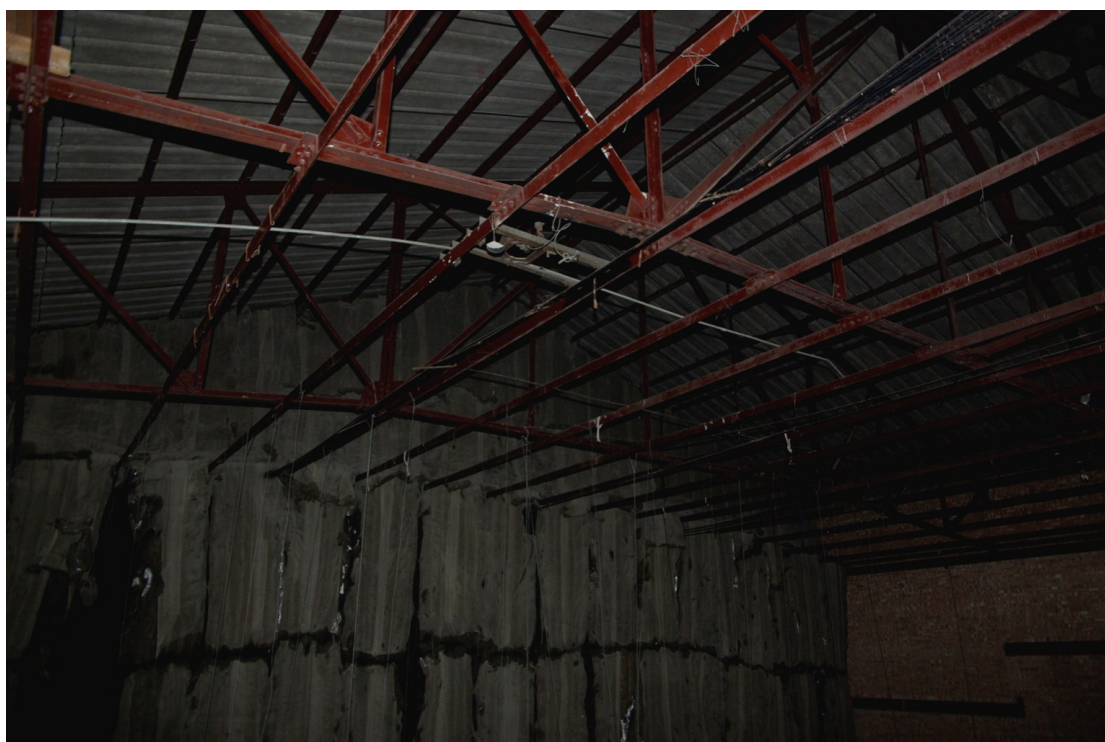
Figure 25. Roof structure as seen from balcony Looking north-west. Note inserted fire screen.
