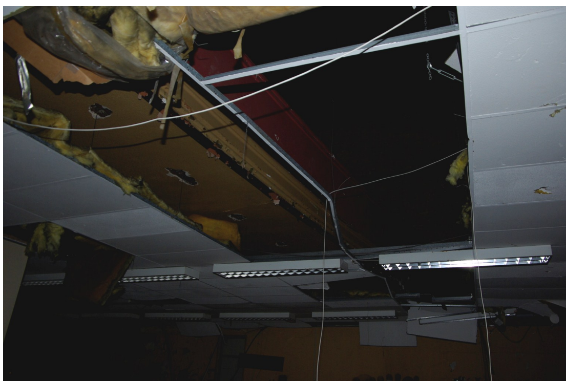
Figure 19. Front and underside of balcony seen through modern false ceiling Looking south-east
