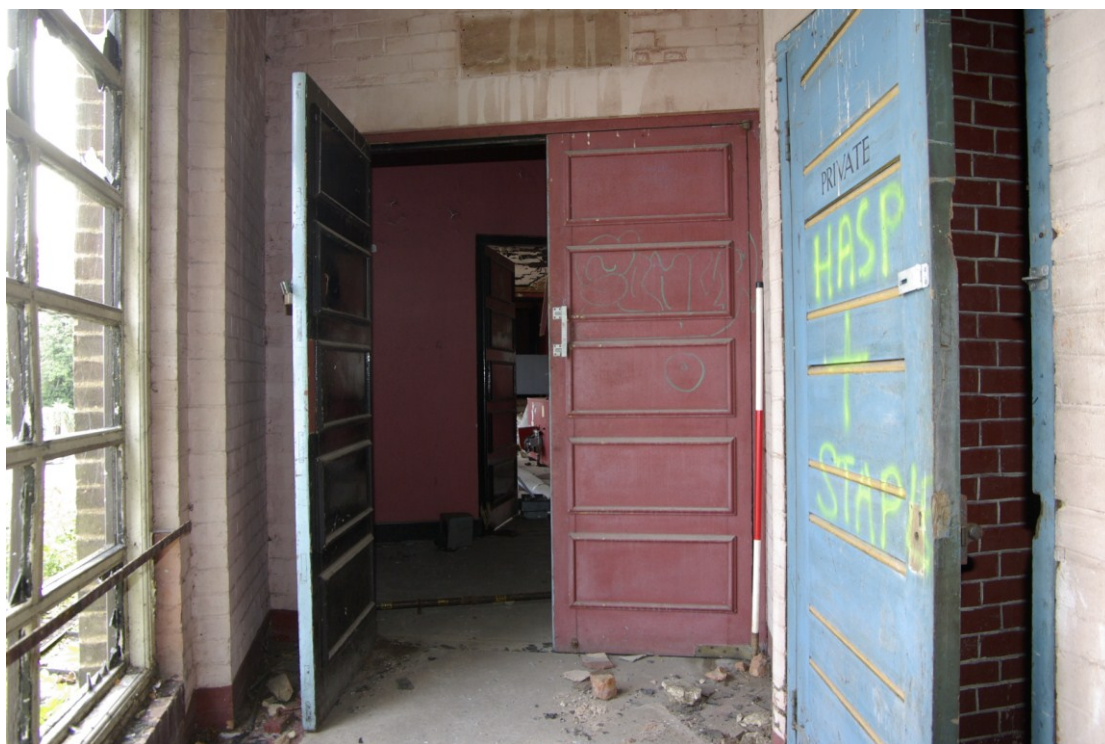
Figure 23. Door details on north side of first floor landing Looking south. 1.5m scale
