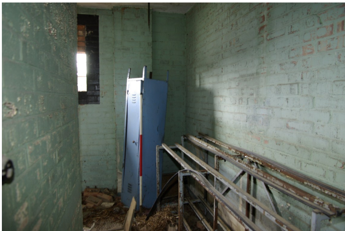
Figure 28. Battery Room Looking west. 1.5m scale
