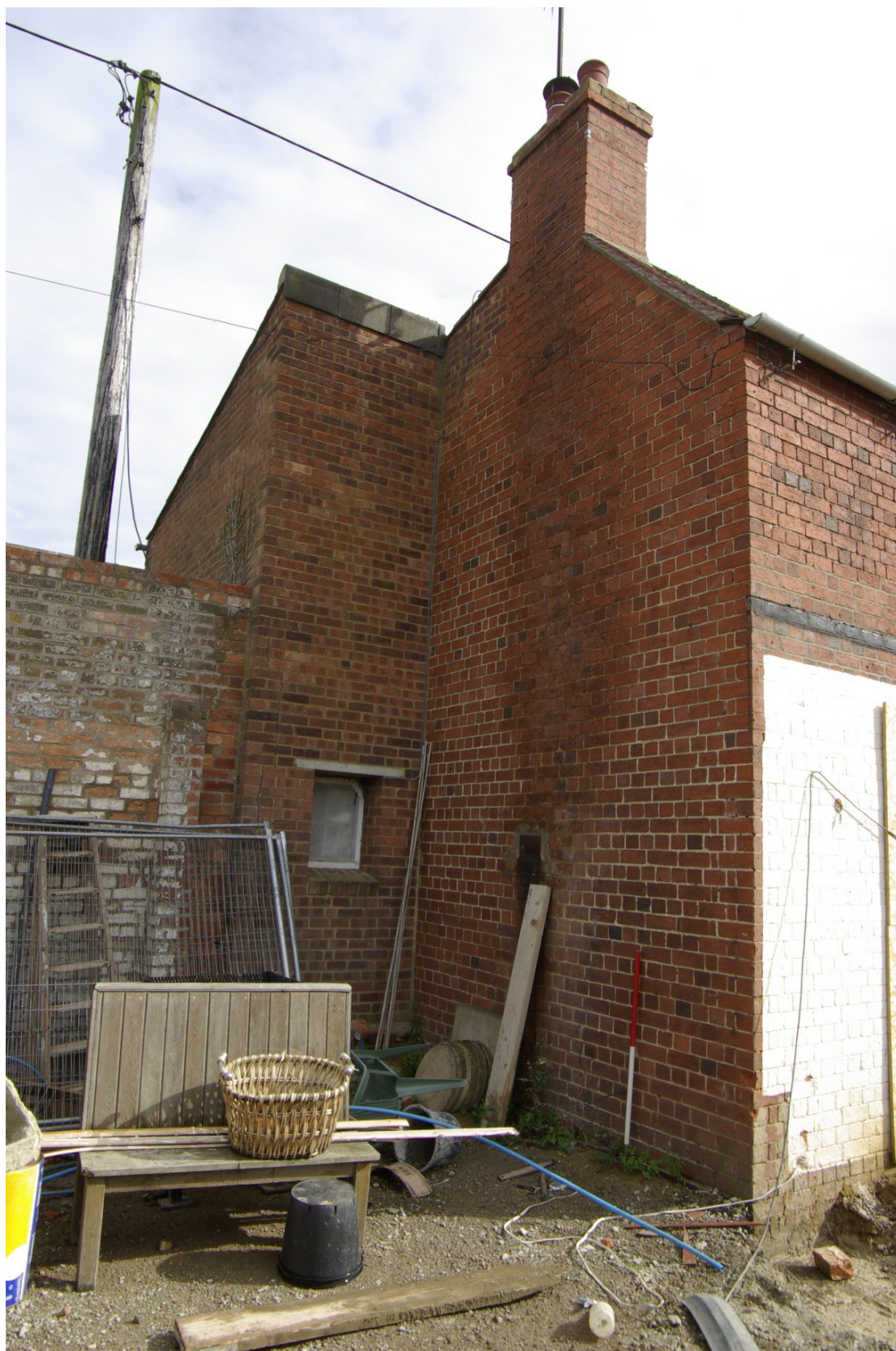
Figure 11. North-west facing elevation to south of garden wall Looking east. 1m scale
