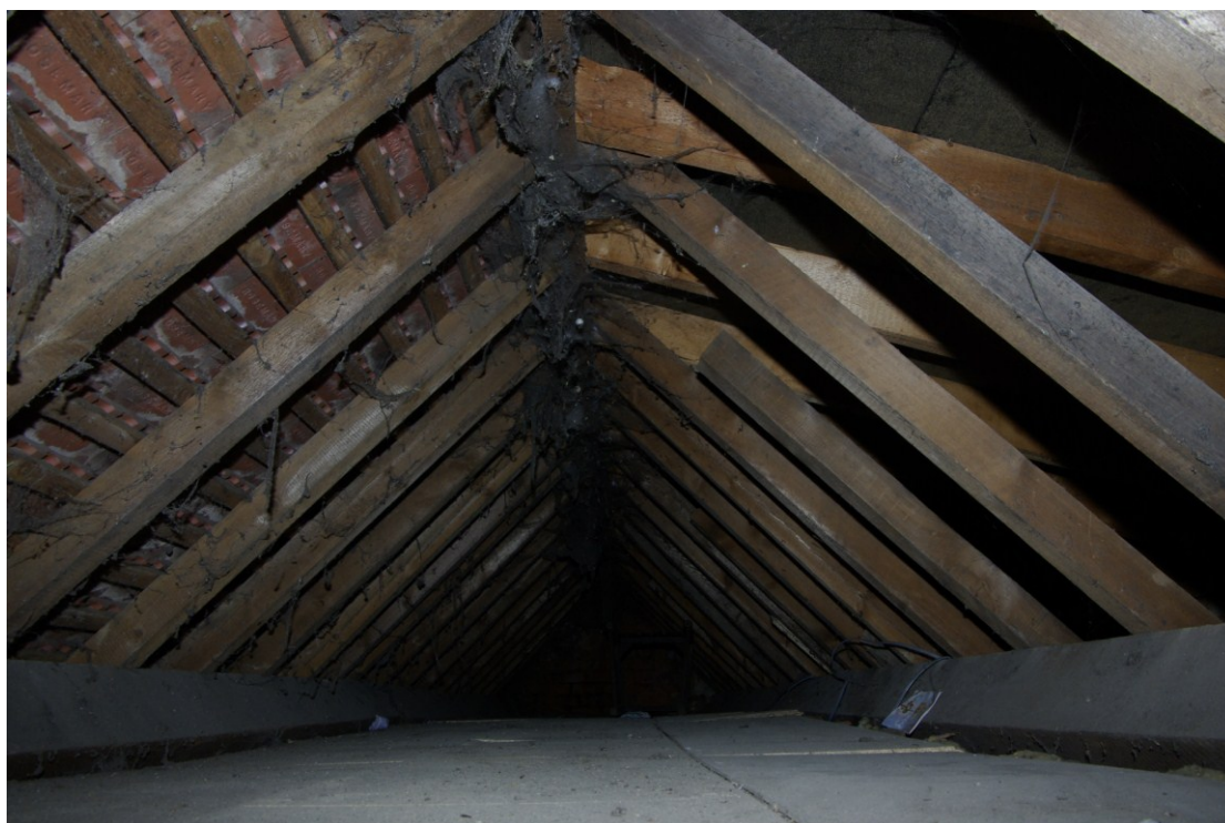
Figure 21. Roof structure Looking north-west. Original phase on left, later extension roof on right
