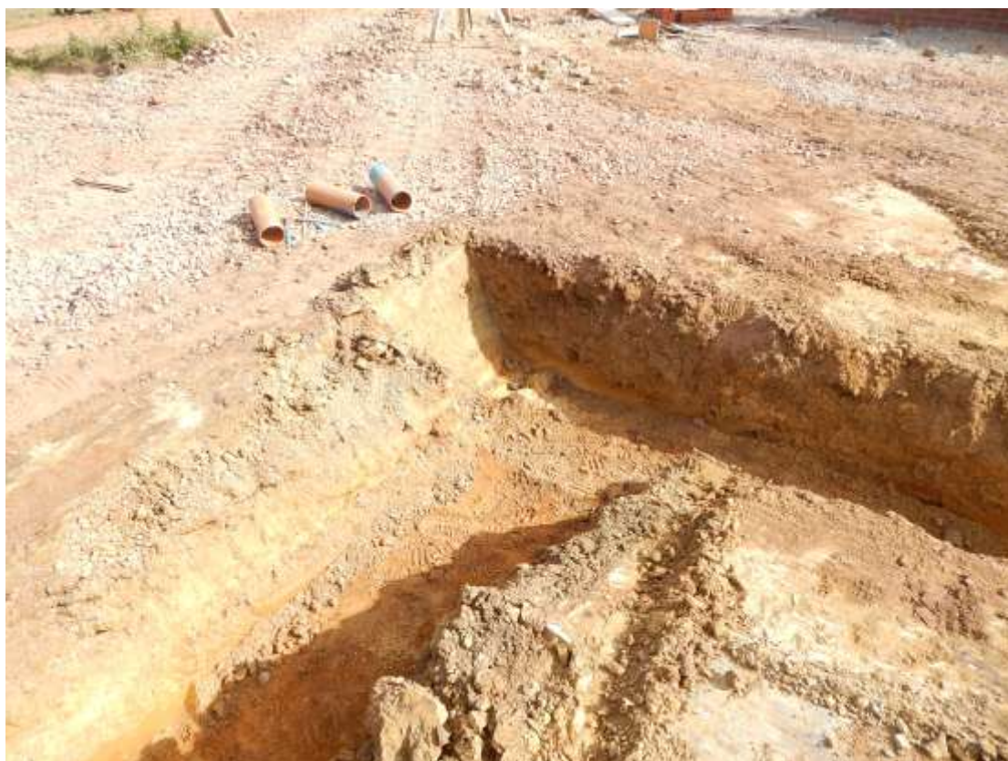
Figure 44: Excavated foundation trenches, Plot 90, showing lack of upper soils, looking north-east
